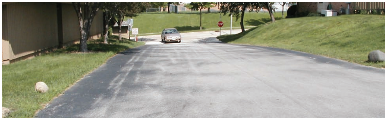
Gray asphalt pavement shows through where sealcoat has worn off the driveway of an apartment complex.
