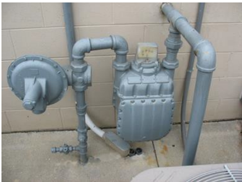
NATURAL GAS EMERGENCIES
