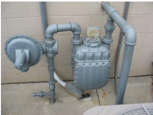
NATURAL GAS EMERGENCIES
