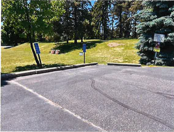
This photo shows an area with accessible signs but missing striping and a van access aisle.
