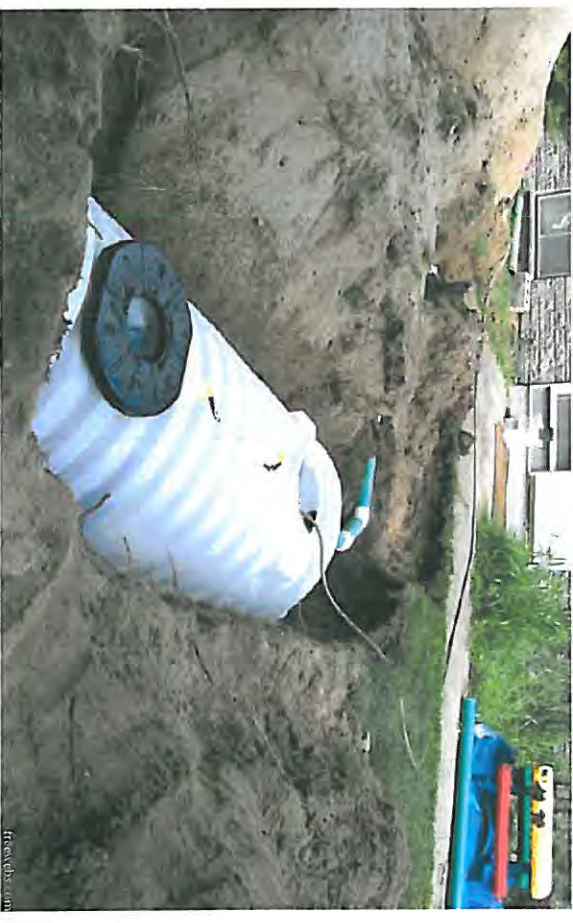
Higher densities increase the amount of septic tanks and effluent within the ecosystem.
