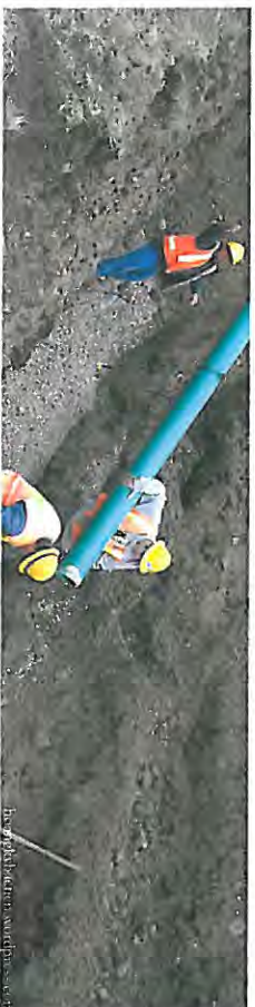
Sewer systems are sized over capacity to allow for higher densities, growth, and more users.
