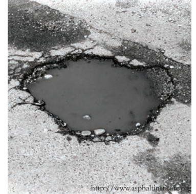
Patches and Potholes
