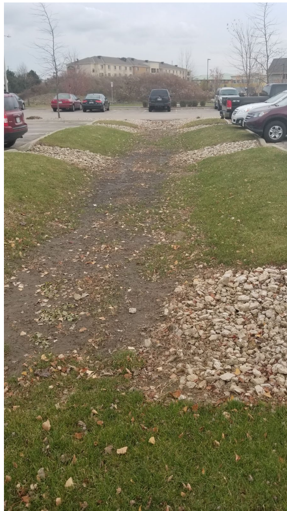
Infiltration area in use for 4 years (Note sediment build-up)
