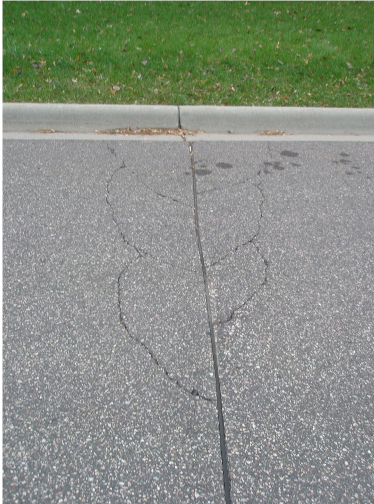
Deer Pond Court 2018 (4 years old) Random cracking. Sinking pavement.
