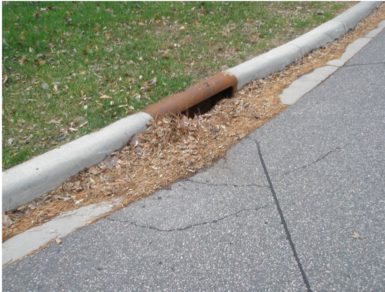
Deer Pond Trail & Court Intersection 2018 (4 years old) Debris on catch basin. Random cracking not sealed.
