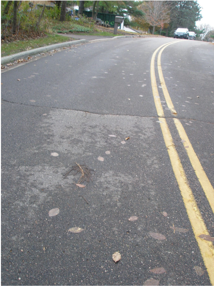
Deer Pond Trail 2018 (4-year old pavement) Looking Uphill Random crack is not sealed.
