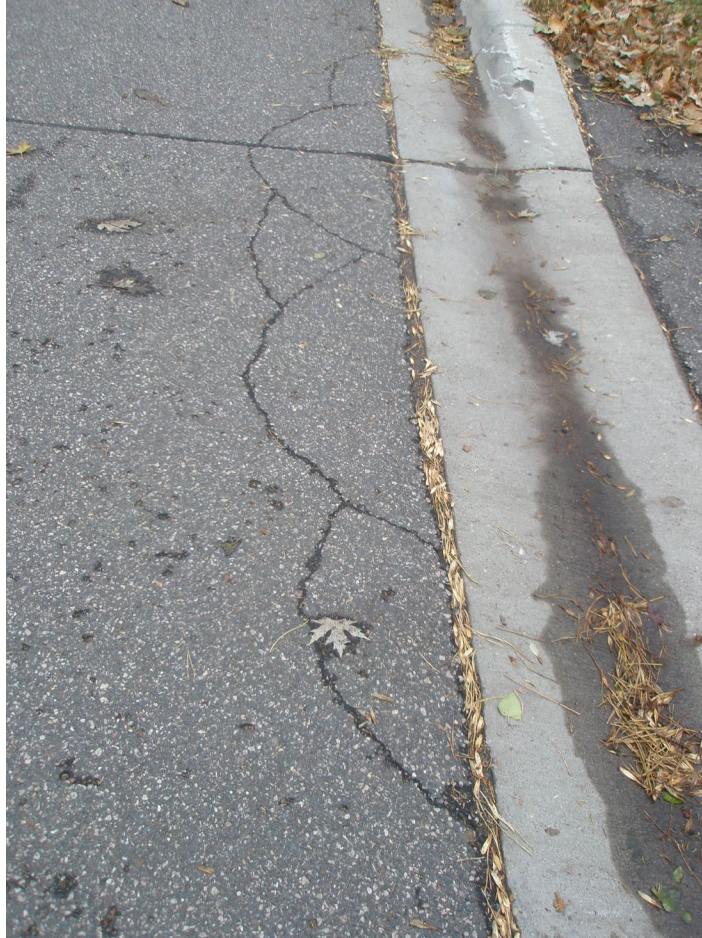
Deer Pond Court 2018 (4-years old) Random Bituminous Cracking Along Concrete Curb
