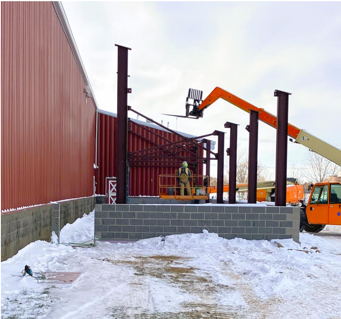
The majority of the concrete in the Fire Department apparatus bay has been poured. The front of the new addition that will house the main entrance, City
