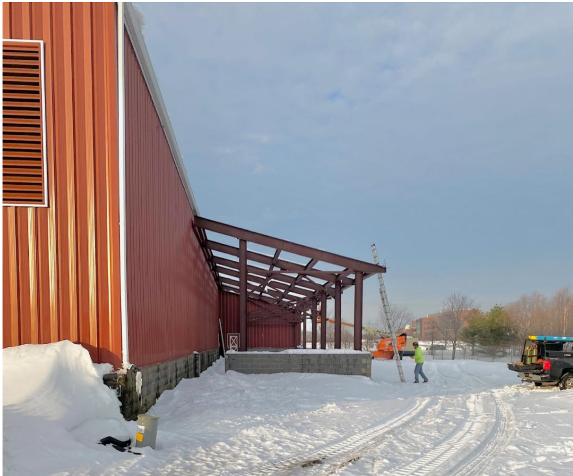
The addition to the public works building on Ideal Avenue is taking shape after delays in delivery of steel for several weeks.
