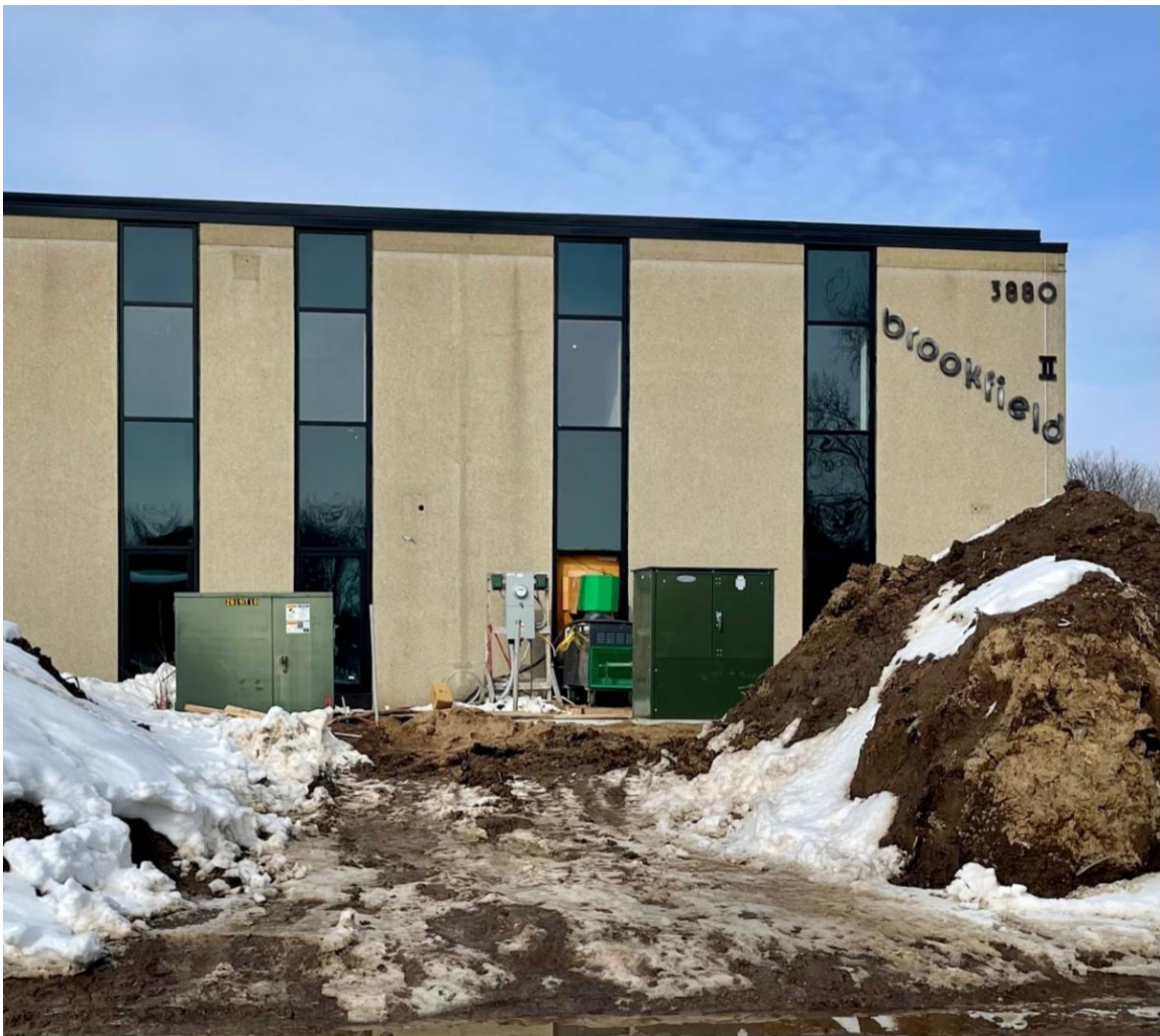
Preparations were made this week for the electric transformer that should arrive next week.
