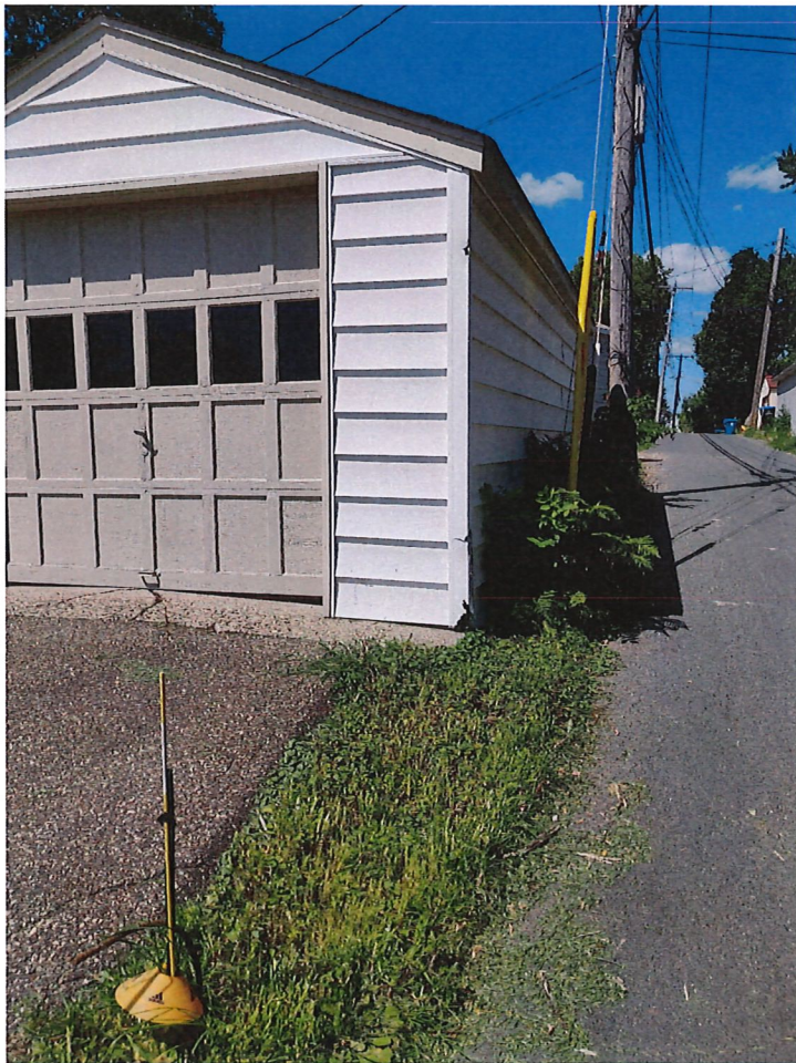
Damage to siding from garbage and recycling trucks
