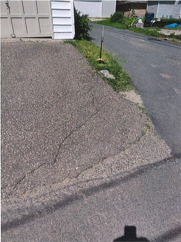
Damage to pavement from garbage and recycling vehicles
