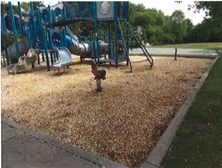
In the above photo, the wood chips are too low and the concrete curb bars access to persons with disabilities. These were common issues in all our cities.
