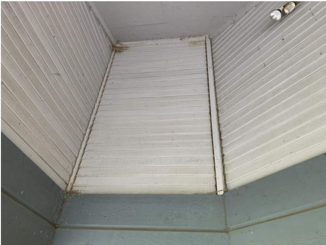
Figure 32 – S28: SW Side (Caulking)
