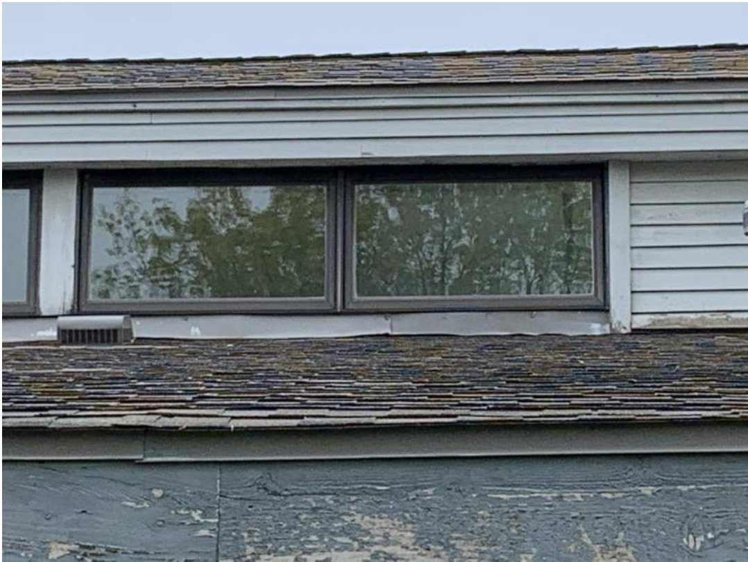
Figure 65 - S61: NE Side (Flashing Deflections)
