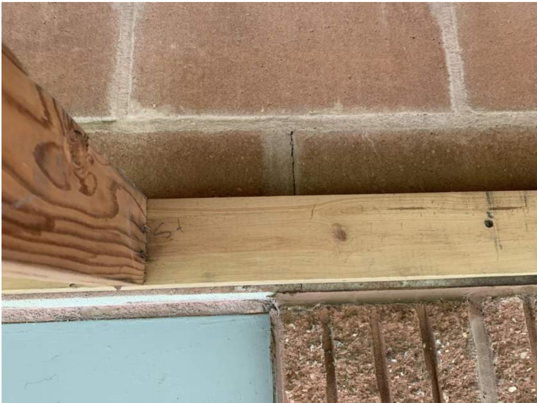
Figure 56 - S50: NE Side (Crack Above Women's Restroom)
