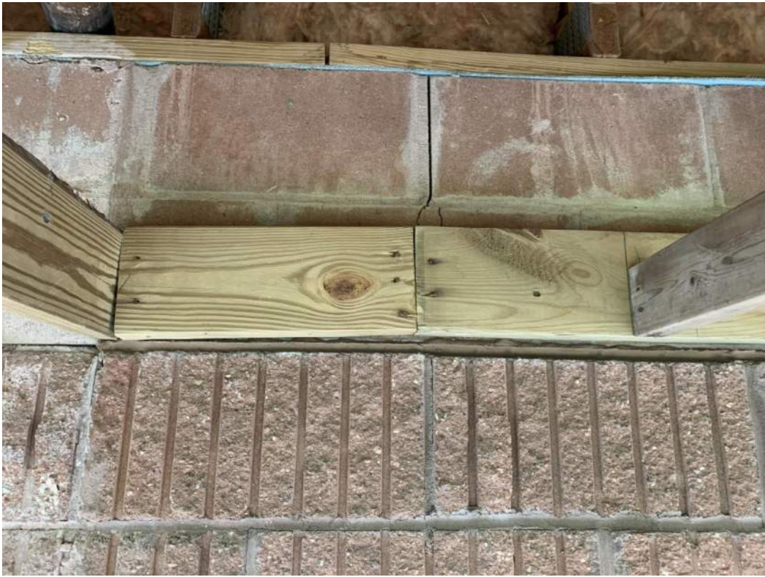
Figure 59 - S53: NE Side (Crack)
