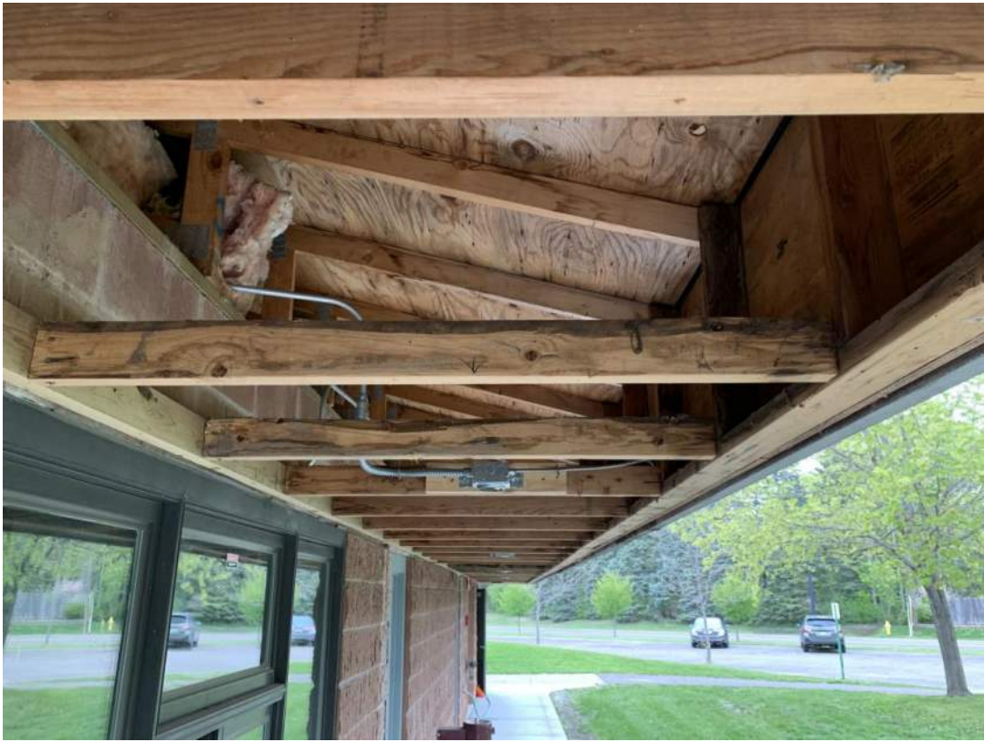
Figure 53 – S47: NE Side (Soffit Missing)
