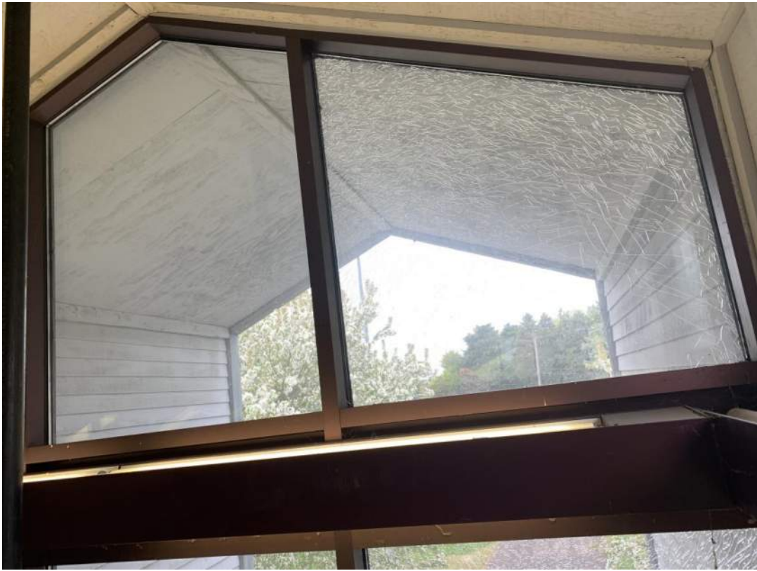
Figure 89 - N13: SW Side (Shattered Windows)
