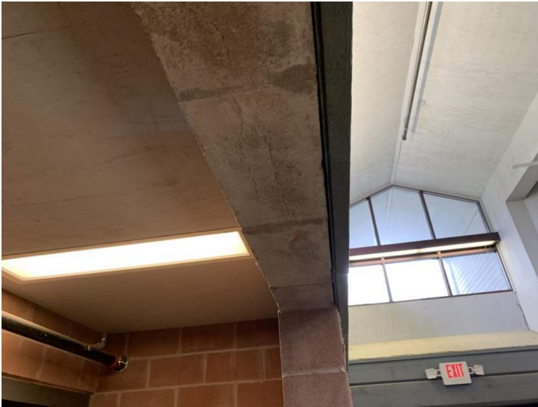
Figure 73 - S69: Main Room (Lintel Crack)
