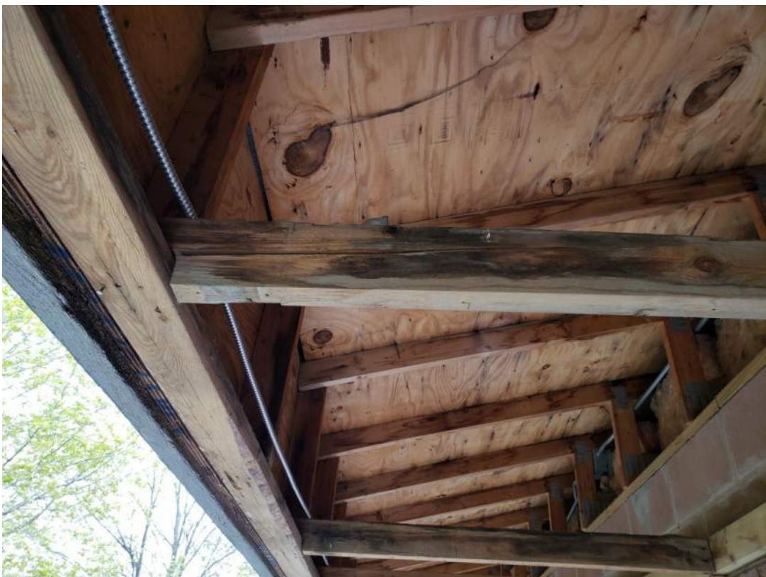
Figure 58 - S52: NE Side (Cracked Joist)
