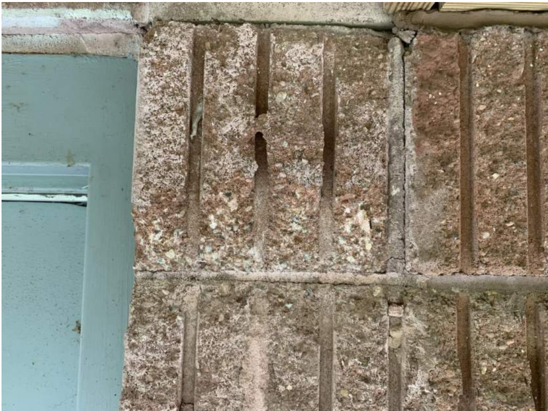
Figure 66 - S62: NE Side (Step Cracking)
