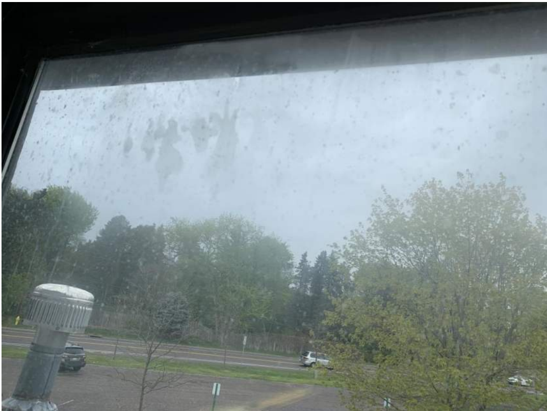
Figure 100 – N24: Interior Main Room (Windowpane Moisture)
