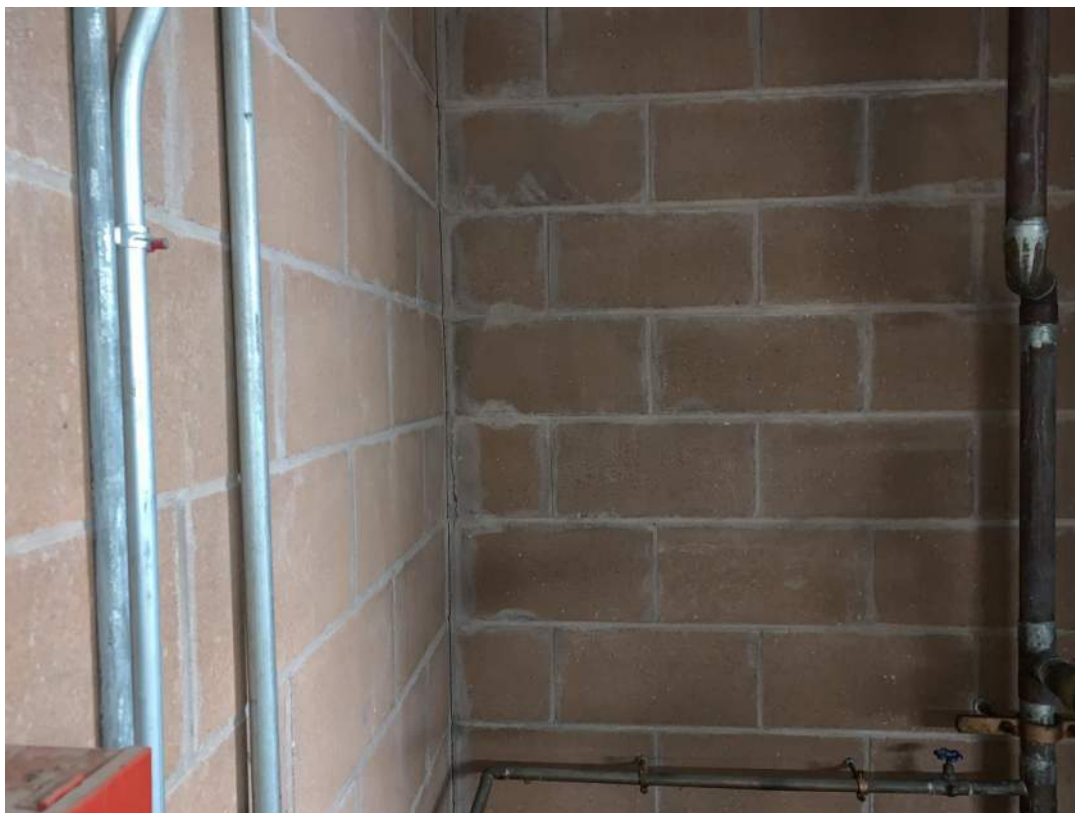
Figure 68 - S64: Storage Room (Wall Gap)
