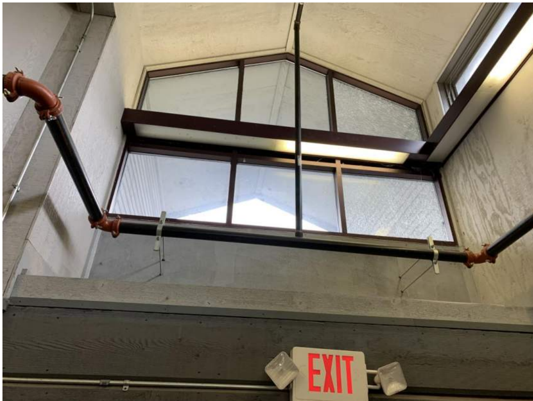
Figure 95 – N19: Interior Main Room (Shattered Windows)
