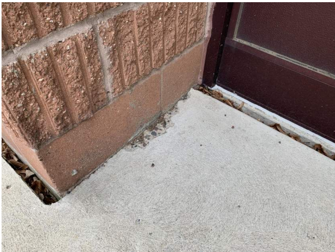
Figure 78 – N2: NW Side (Concrete Spalling)
