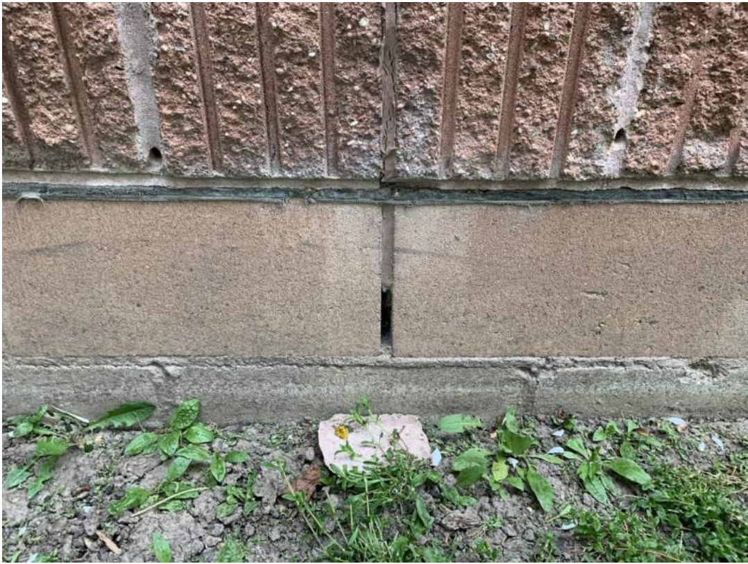
Figure 47 - S42: SE Side (Mortar Breakout)
