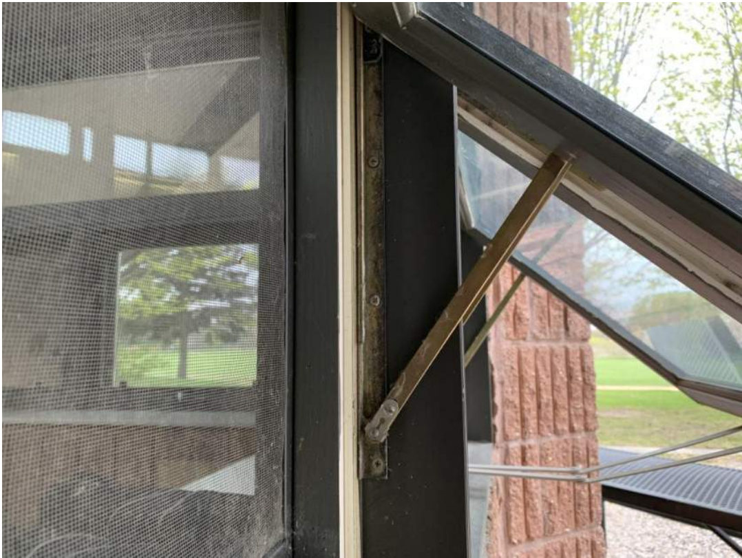
Figure 83 - N7: SW Side (Corrosion on Tracks)
