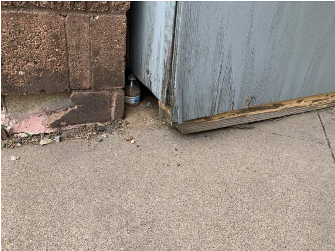
Figure 80 - N4: NW Side (Shed Water Damage)
