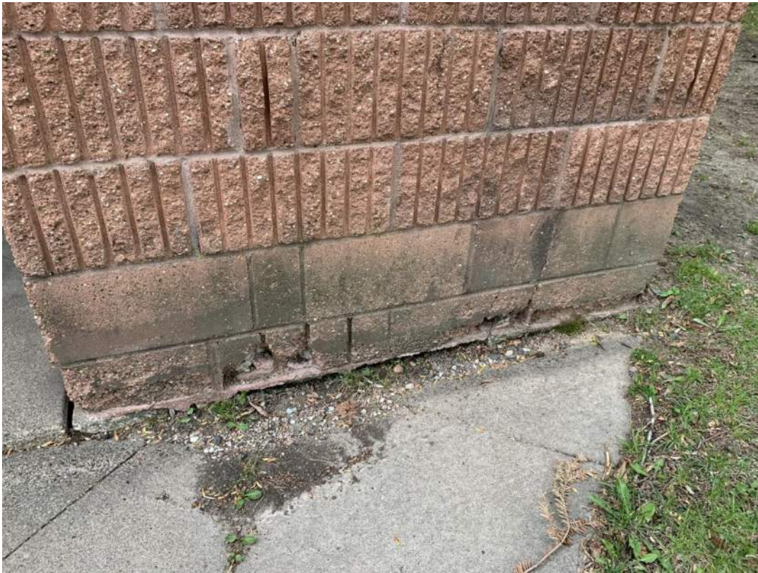
Figure 35 – S31: SW Side (Masonry Breakout)
