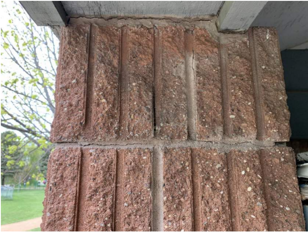
Figure 29 - S25: SW Side (Cracks)
