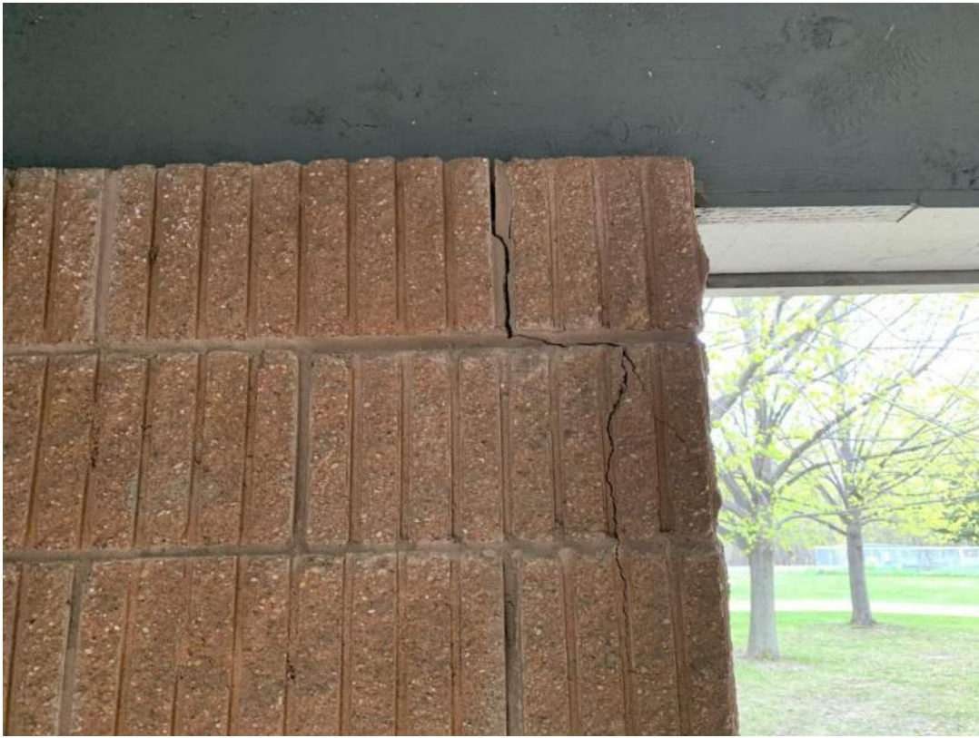
Figure 37 – S33: SW Side (Step Cracking)
