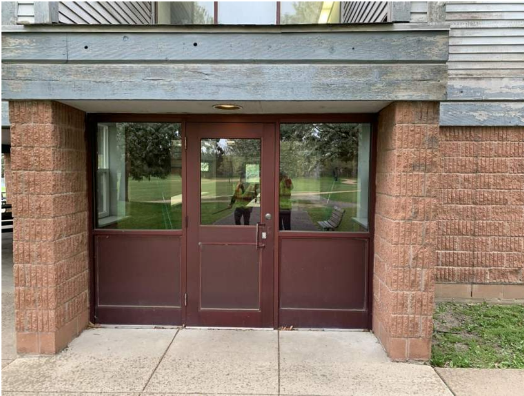
Figure 43 - S39: SE Side (Spalling Left of Door)
