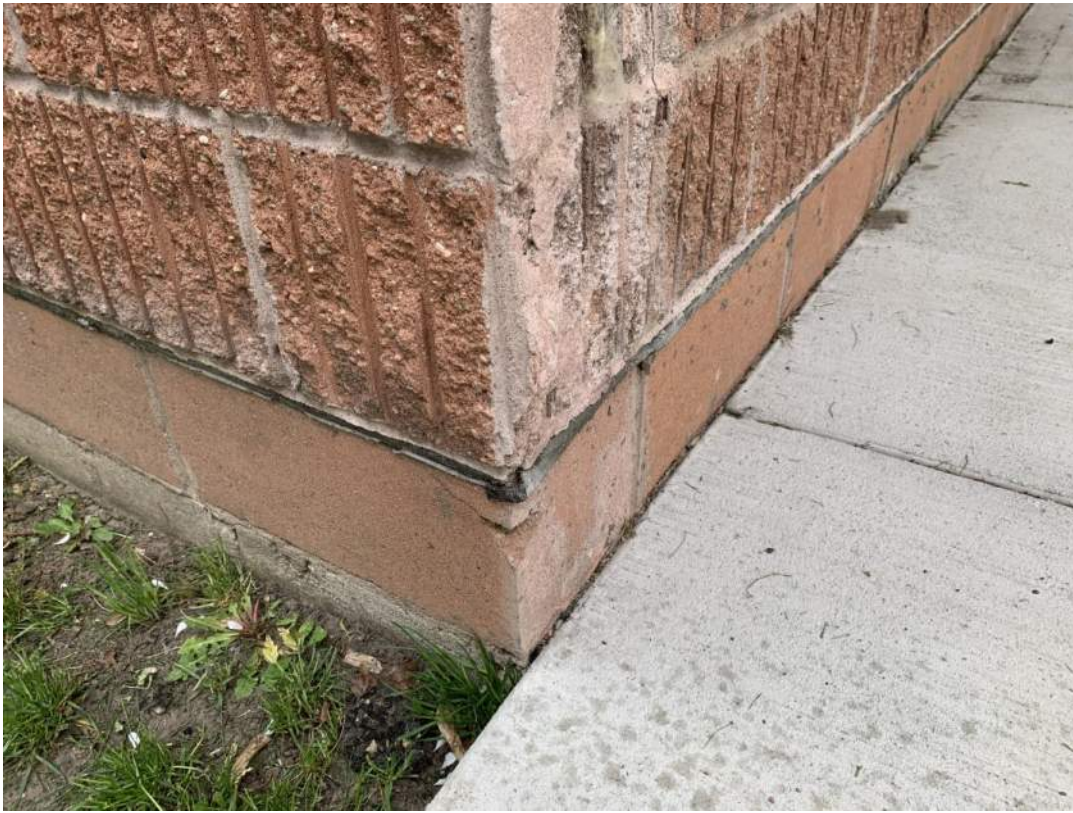
Figure 51 – S45: SE Side (Foundation Crack)
