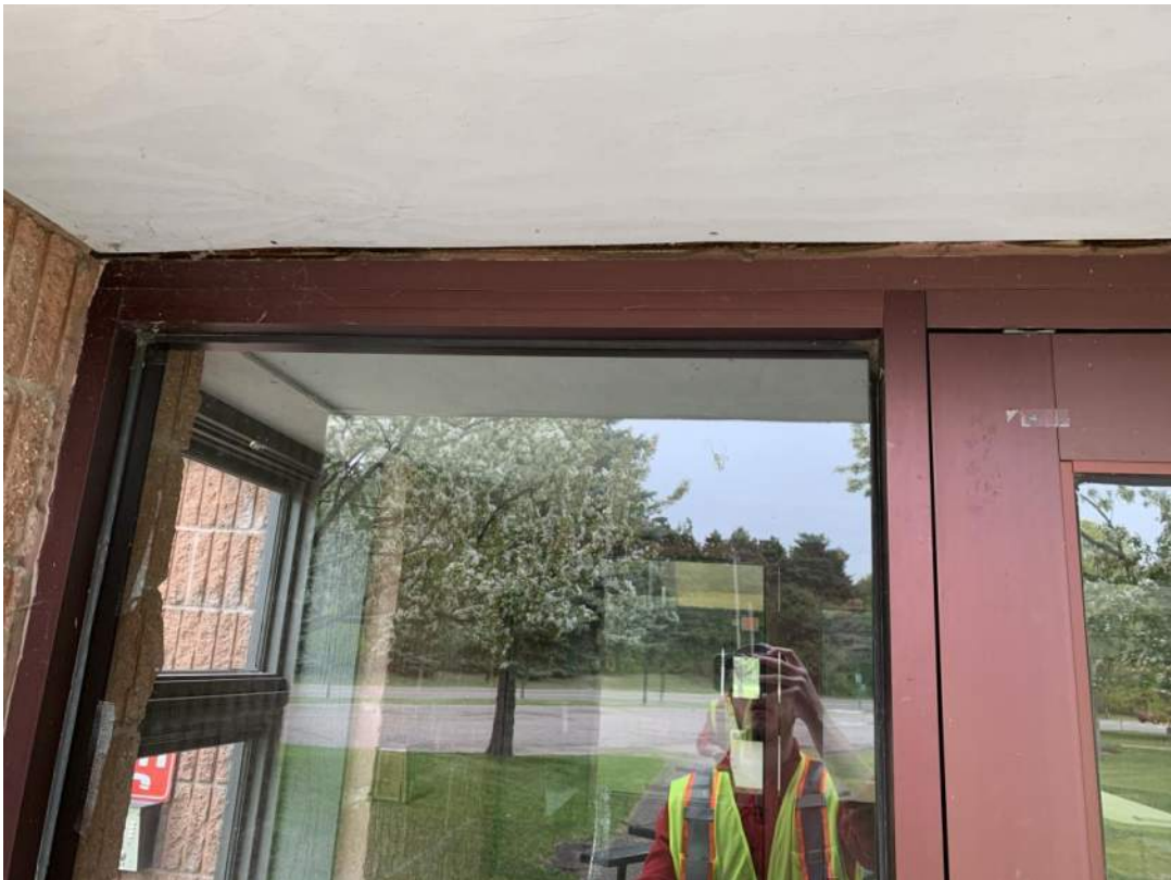
Figure 8 – S1: NW Side (Caulking)
