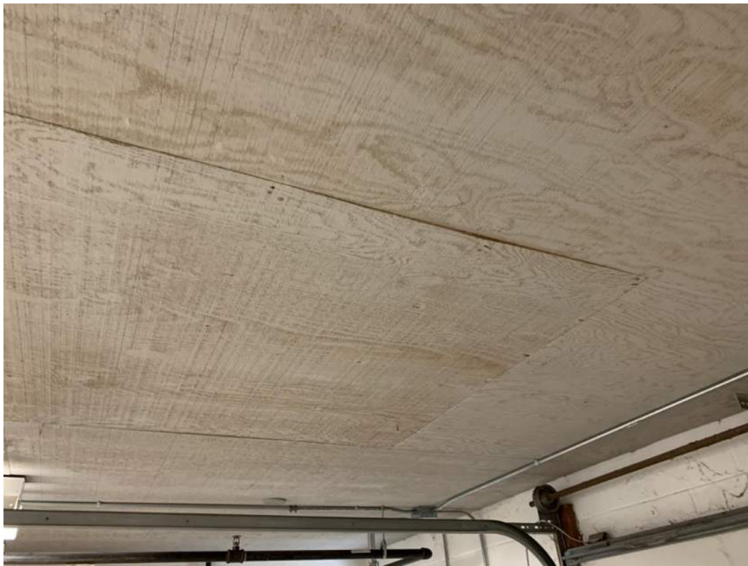
Figure 67 – S63: Storage Room (Ceiling Panel Deflection)
