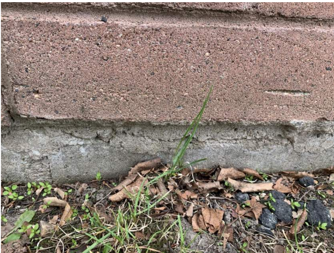
Figure 18 – S12: NW Side (Foundation Crack)
