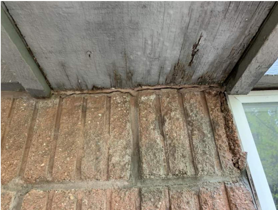
Figure 34 - S30: SW Side (Soffit Water Damage)
