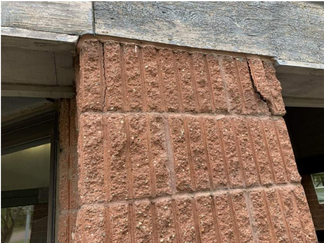
Figure 26 – S21 & S22: SW Side (Exposed Anchor & Masonry Breakout)
