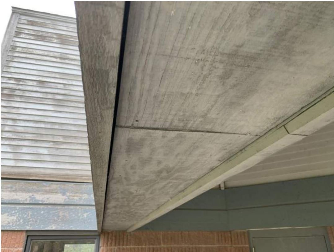
Figure 16 – S10: NW Side (Soffit Deflection)
