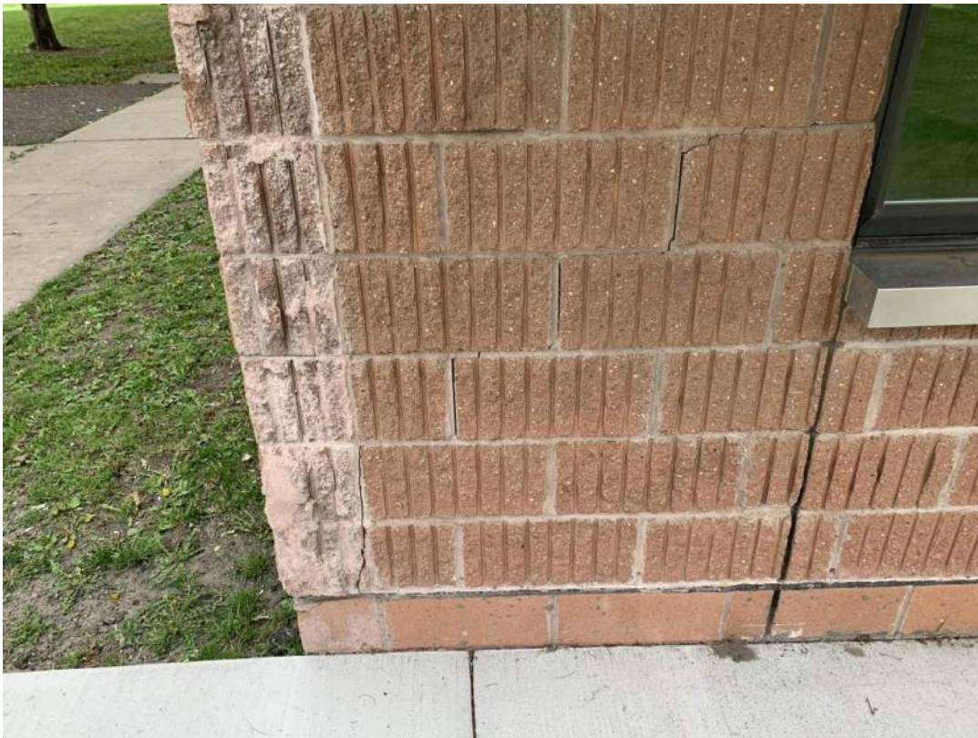
Figure 52 – S46: NE Side (Step Cracking)
