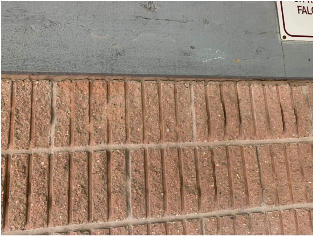
Figure 31 – S27: SW Side (Caulking)
