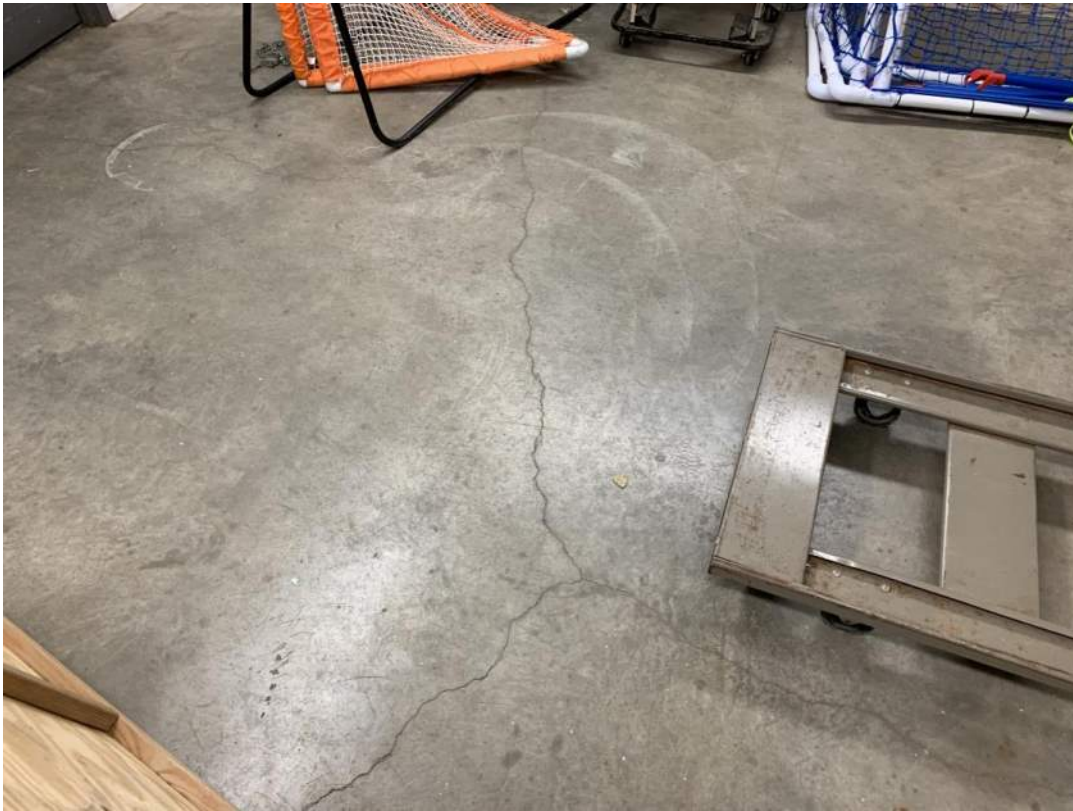
Figure 93 - N17: Storage Room (Concrete Slab Crack)
