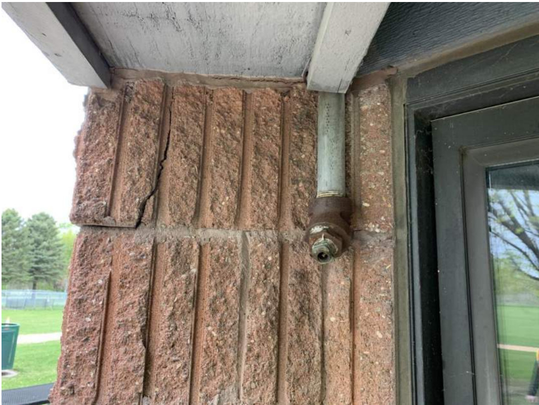
Figure 86 - N10: SW Side (Pipe Corrosion)
