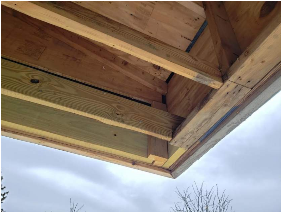
Figure 64 - S59 & S60: NE Side (Loose Joist & Cracked Board)
