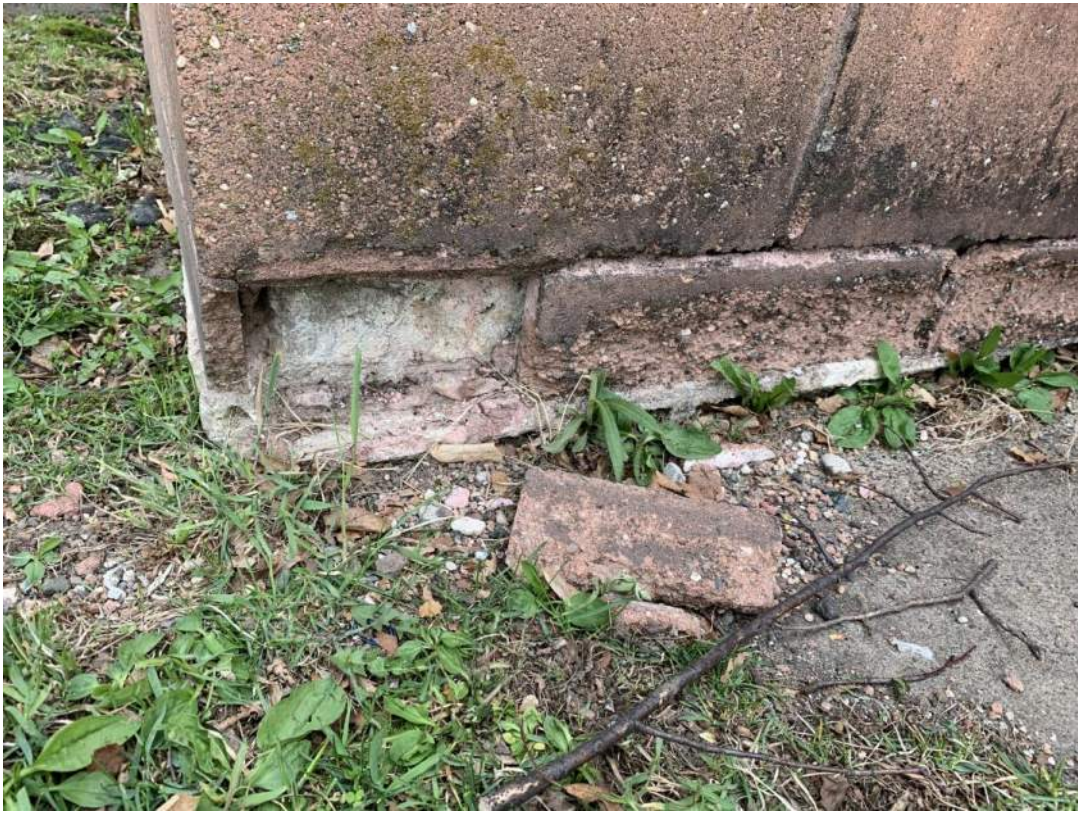
Figure 27 - S23: SW Side (Masonry Breakout)
