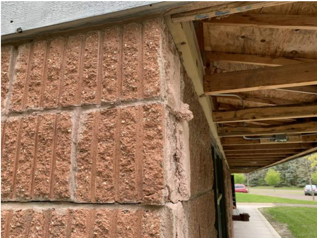
Figure 50 – S44: SE Side (Step Cracking)
