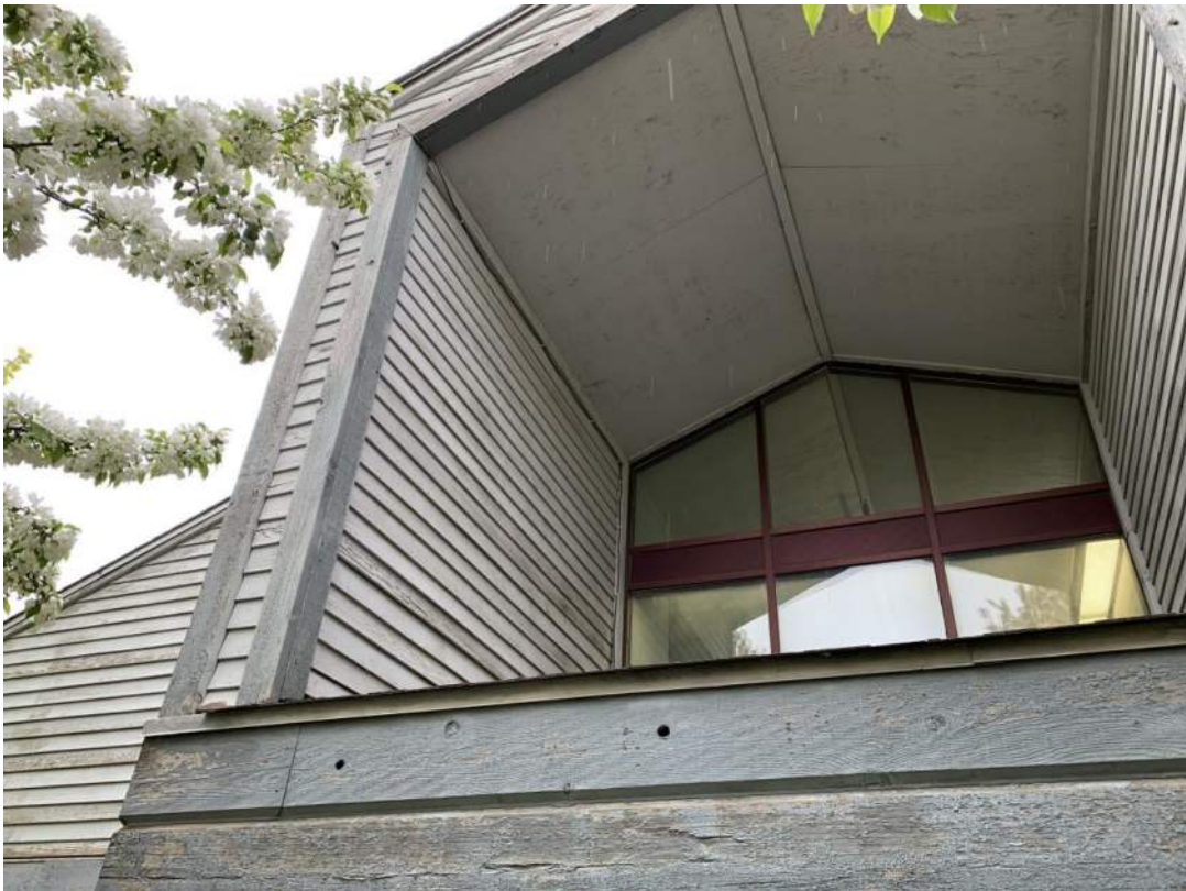
Figure 42 - S38: SE Side (Ceiling Panel Deflection)
