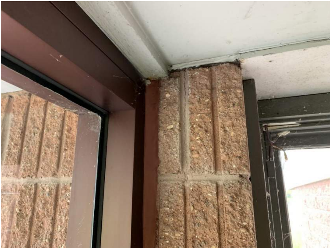
Figure 72 - S67 & S68: Main Room (Caulking & Crack)
