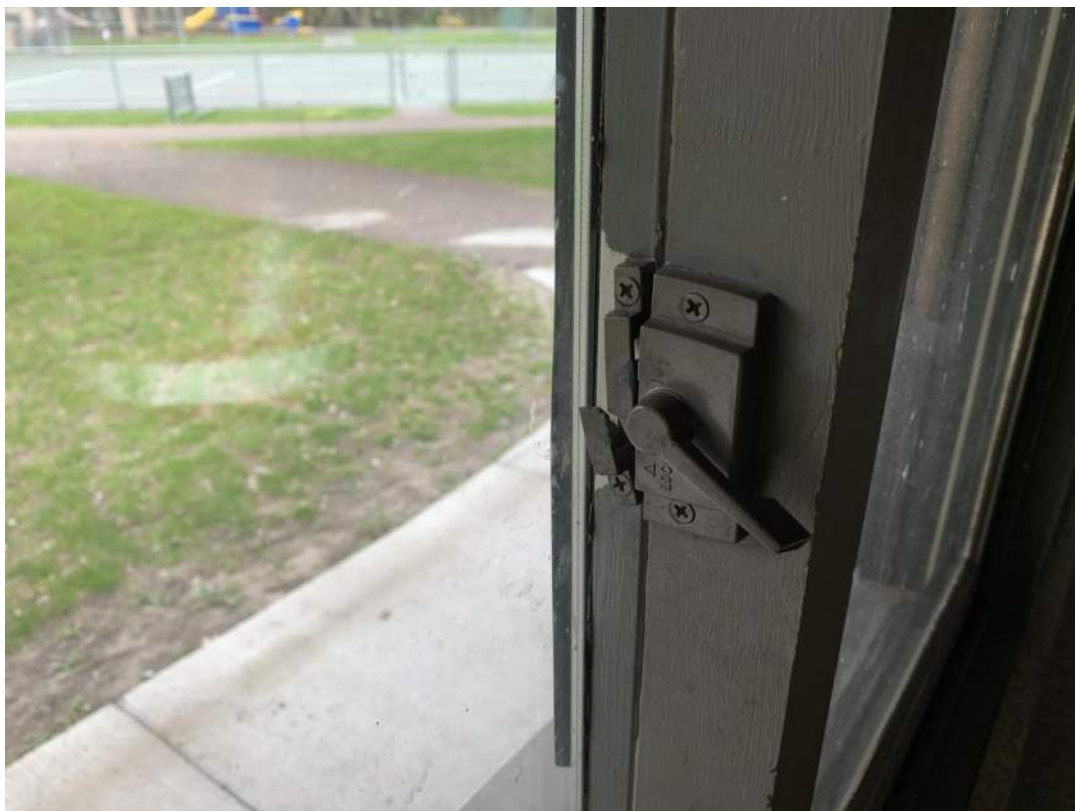
Figure 102 - N26: Kitchen (Window Lock Broken)
