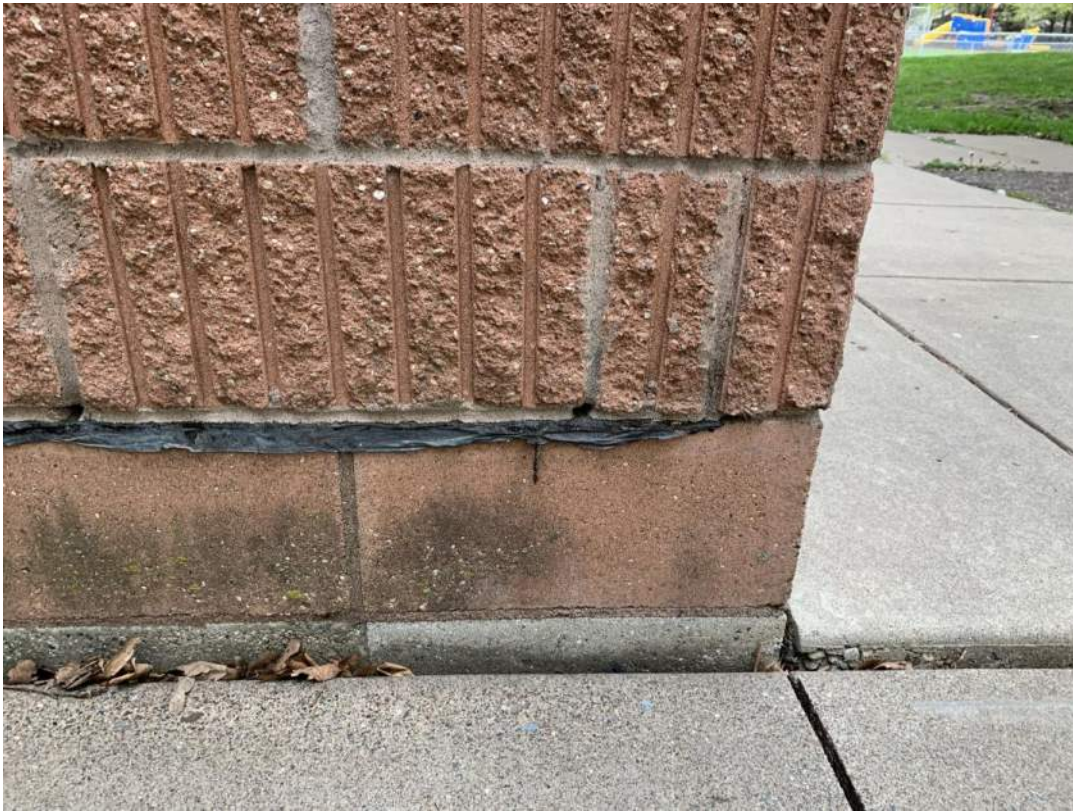
Figure 33 - S29: SW Side (Foundation Cracks)
