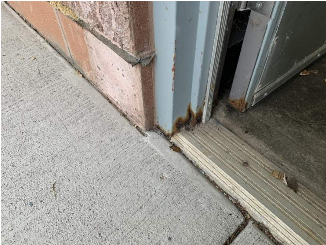
Figure 91 – N15: NE Side (Door Frame Corrosion)
