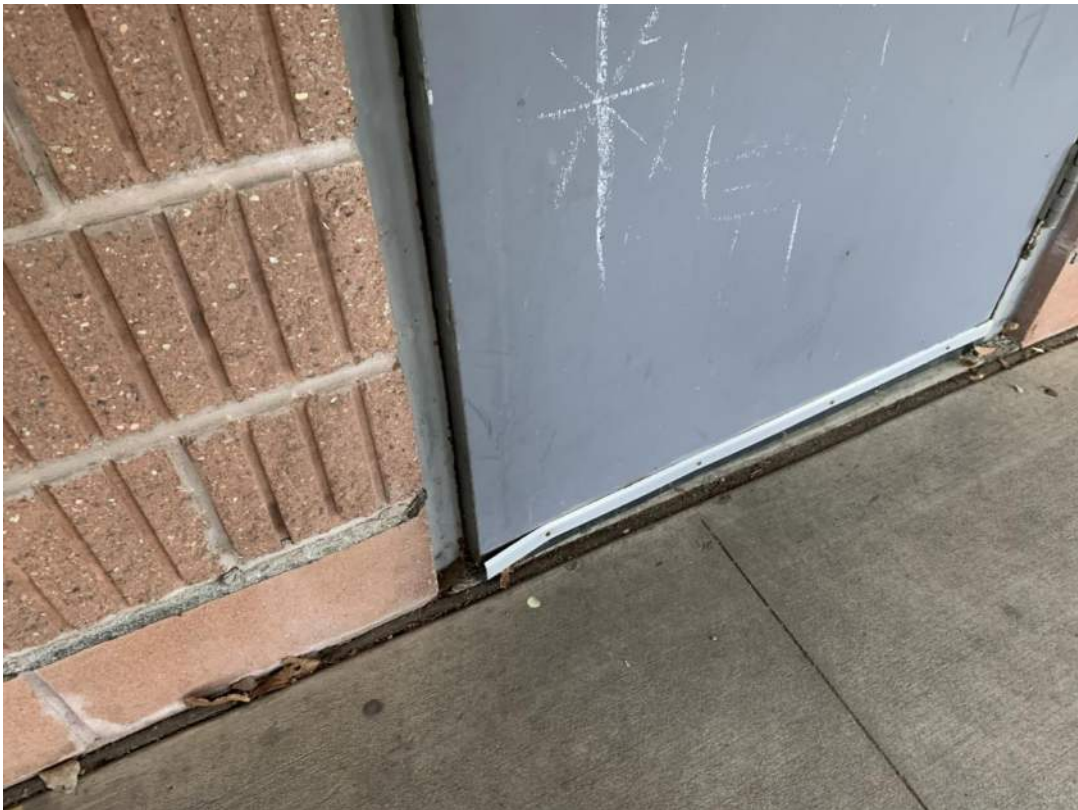
Figure 88 - N12: SW Side (Door Bent)
