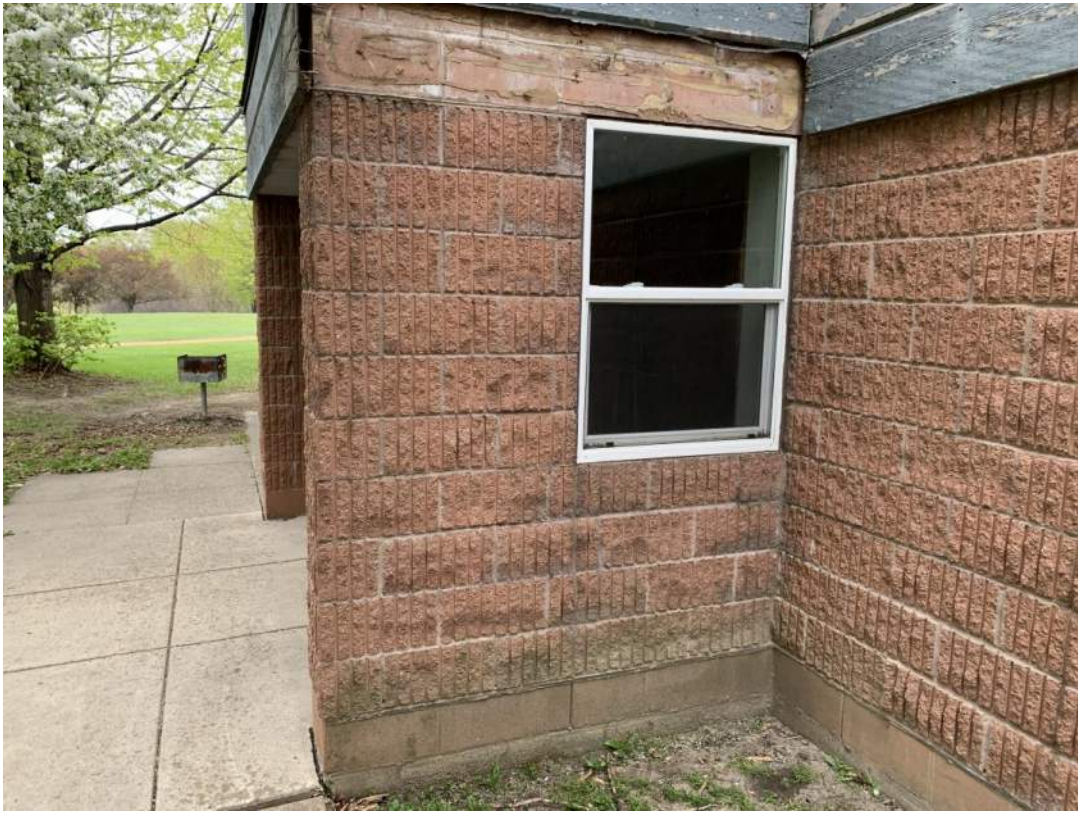
Figure 45 – S41: SE Side (Missing Board & Rotten)
