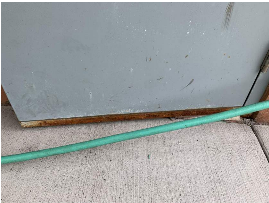
Figure 92 – N16: NE Side (Storage Room Door Corrosion)
