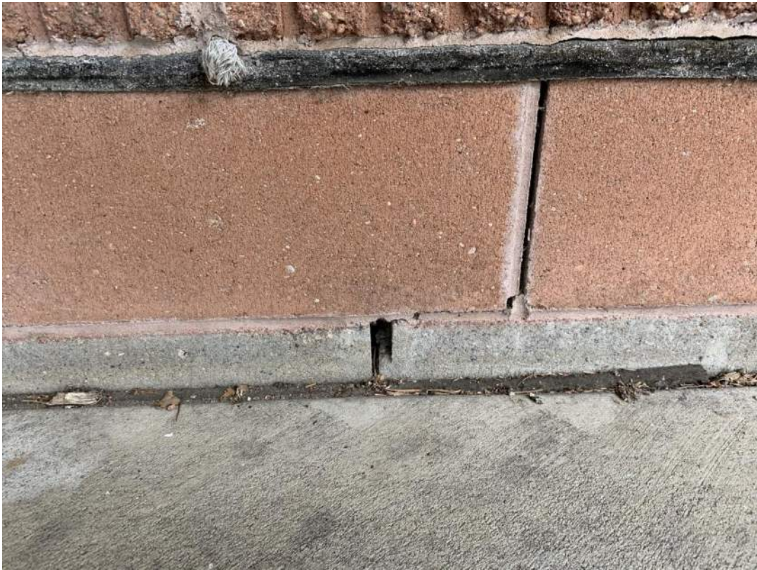
Figure 21 – S16: SW Side (Broken Mortar & Step Crack)
