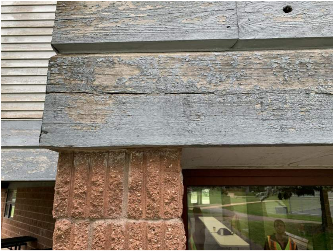
Figure 41 - S37: SE Side (Cracked Trim Board)
