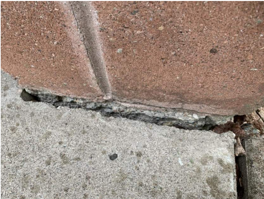
Figure 44 - S40: SE Side (Crack at Foundation)
