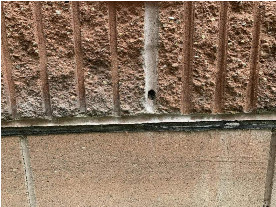
Figure 48 - S43: SE Side (Weep Holes Plugged)
