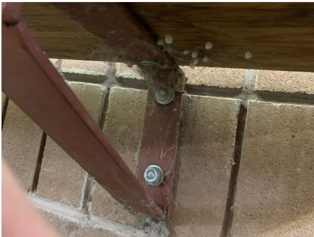
Figure 96 – N20: Interior Main Room (Bench Loose Bolts)
