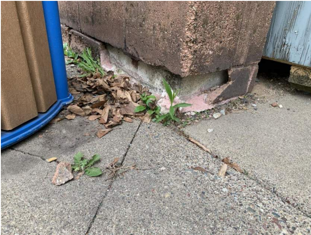
Figure 17 – S11: NW Side (Broken Masonry)
