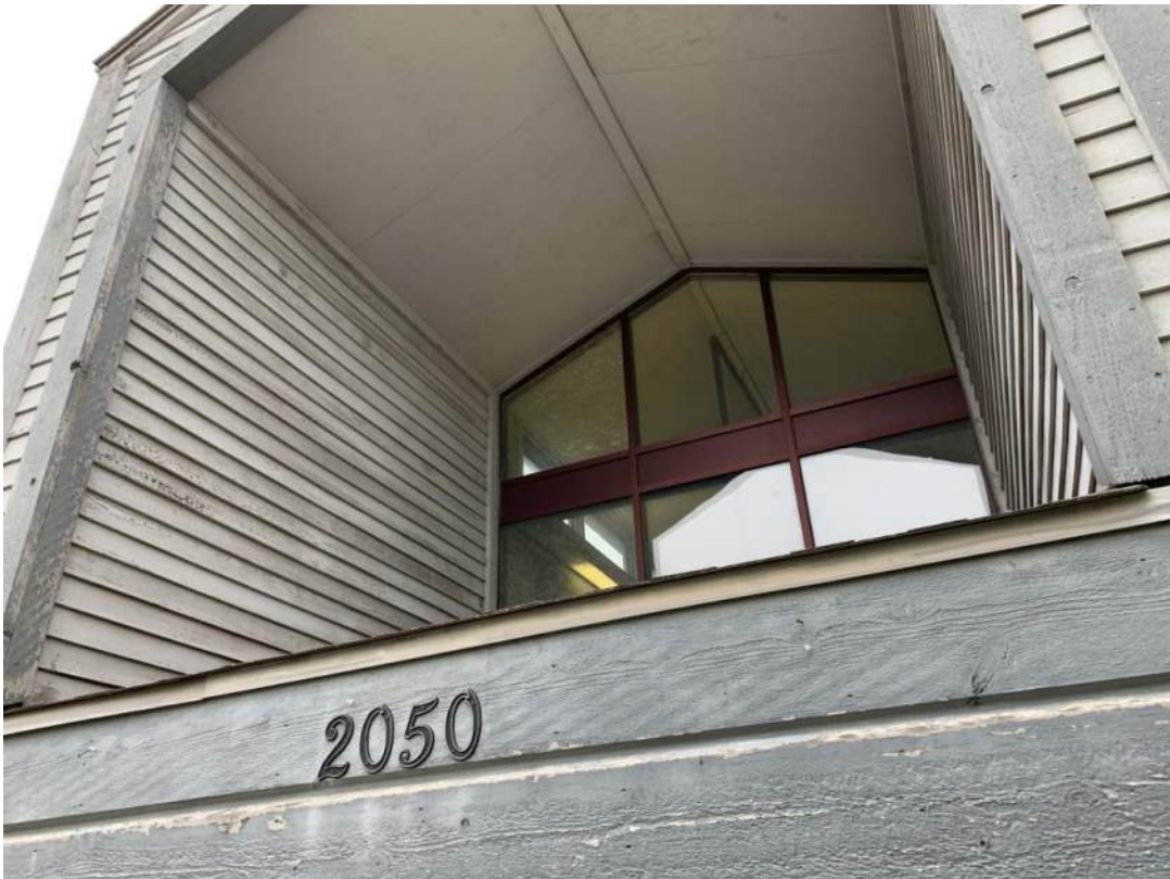
Figure 14 – S6 & S7: NW Side (Panel Deflection & Caulking)
