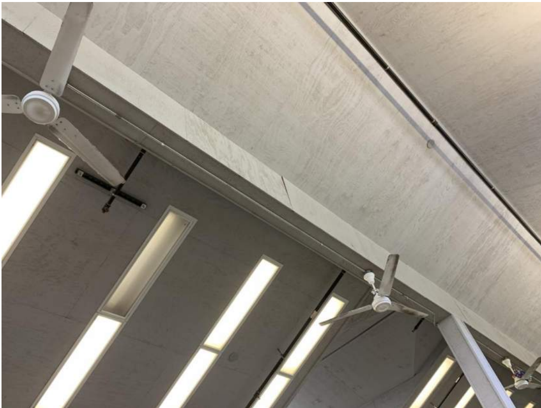
Figure 74 - S70: Main Room (Ceiling Panel Deflection)
