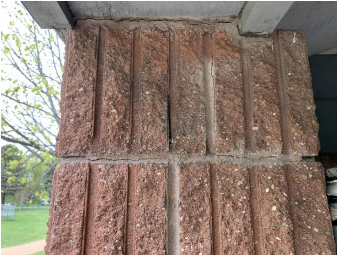
Figure 19 - S13: NW Side (Masonry Crack)
