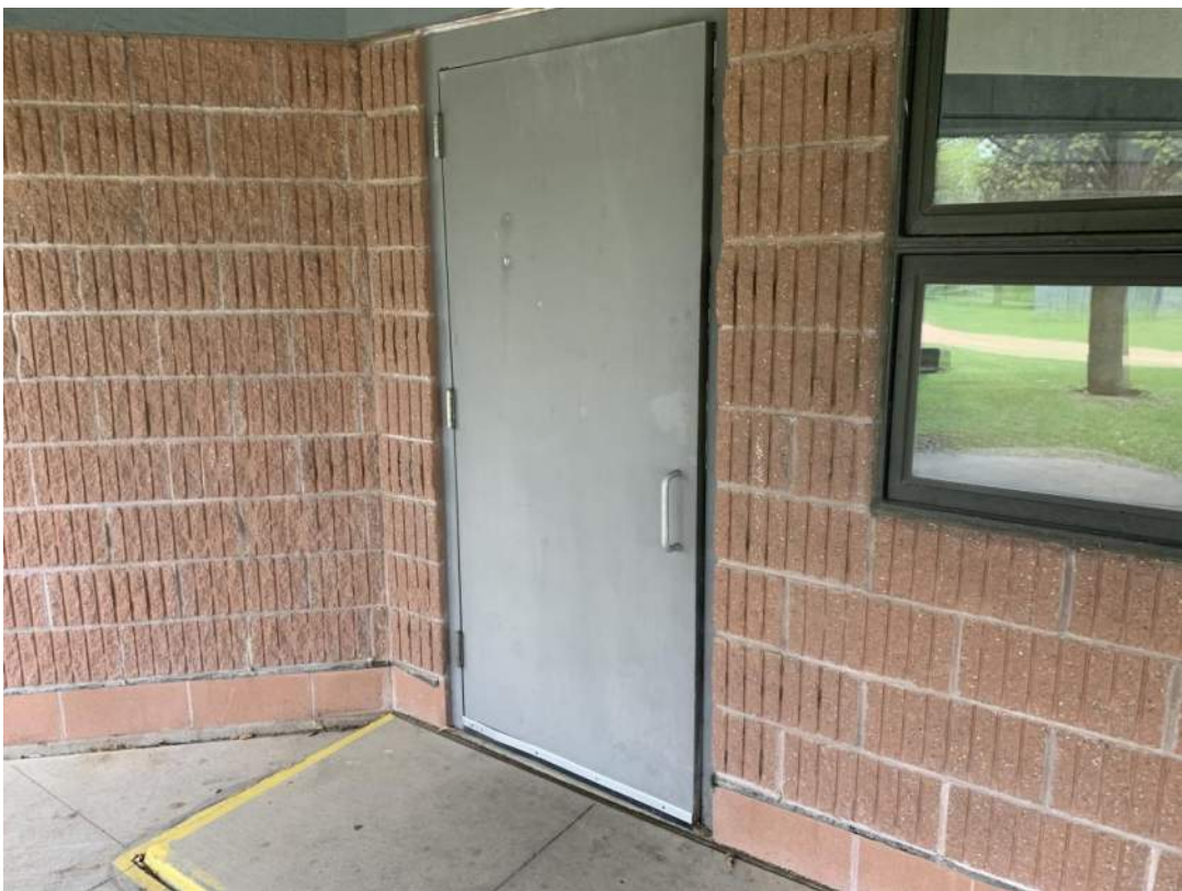
Figure 82 - N6: SW Side (Door Does Not Shut)
