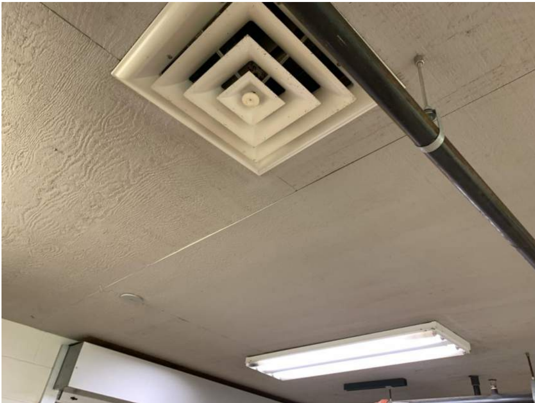
Figure 76 – S72: Kitchen (Ceiling Panel Deflection)
