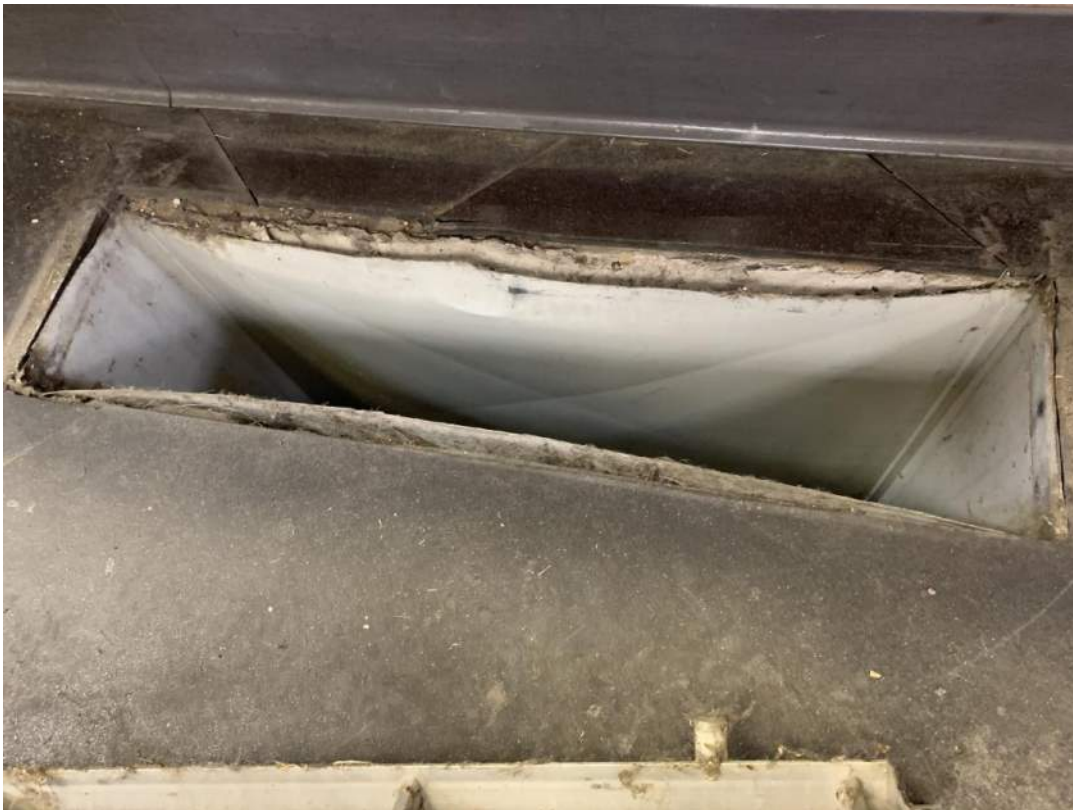
Figure 98 - N22: Interior Main Room (Air Vent Deflections)
