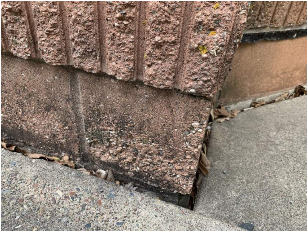
Figure 28 - S24: SW Side (Masonry Spalling)
