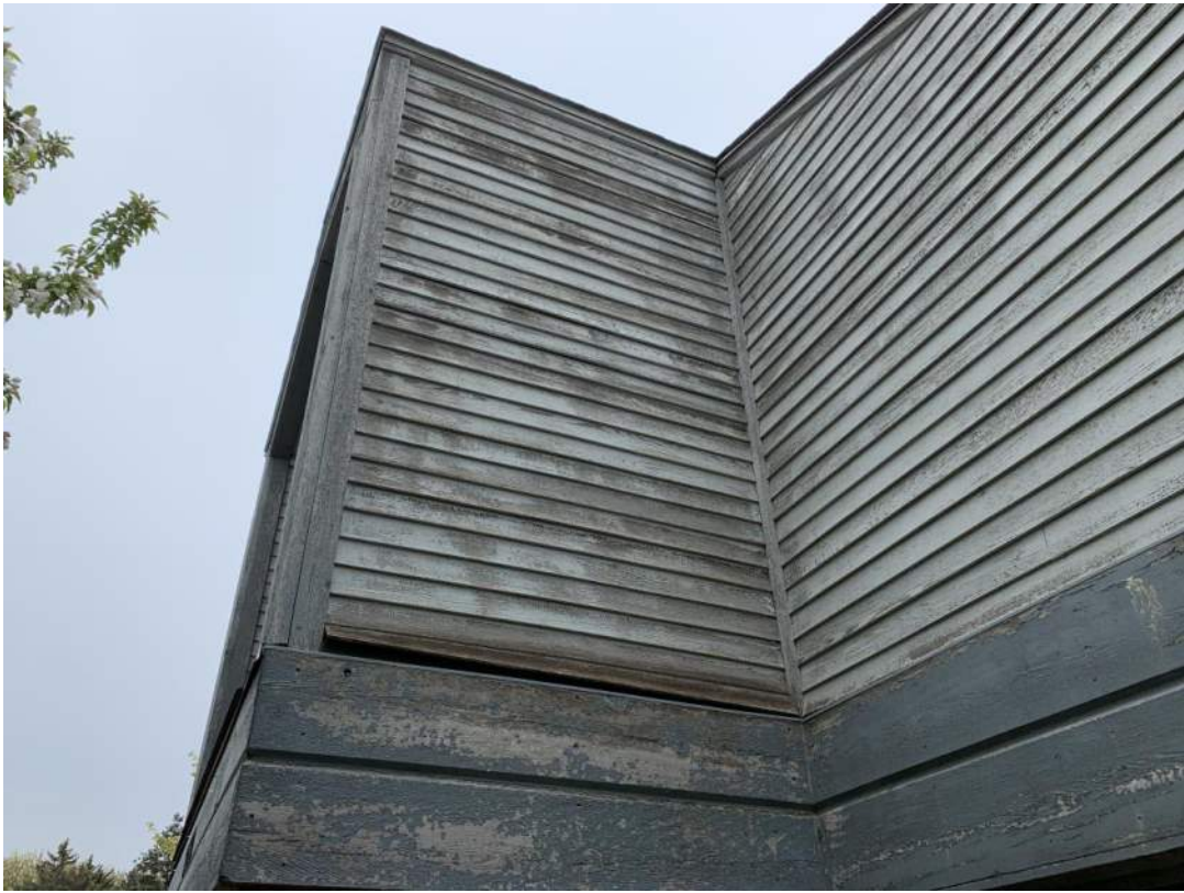
Figure 15 – S8 & S9: NW Side (Caulking & Paint)
