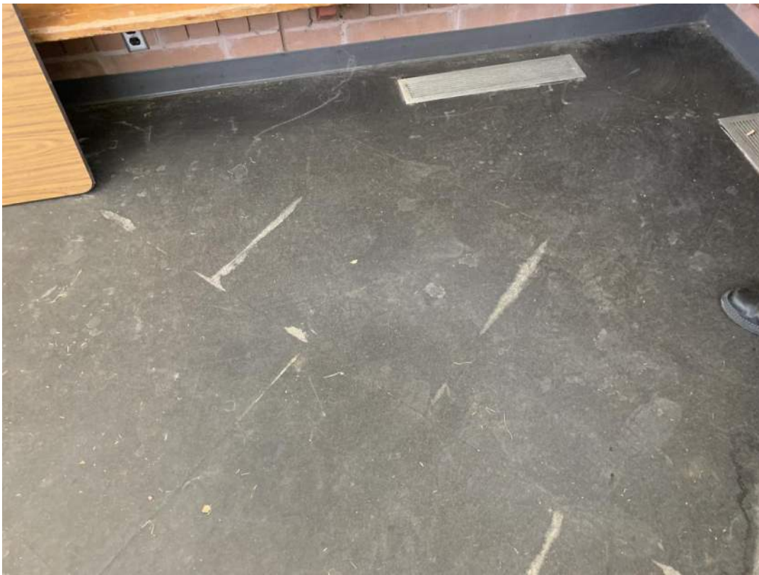
Figure 97 - N21: Interior Main Room (Floor Lump)
