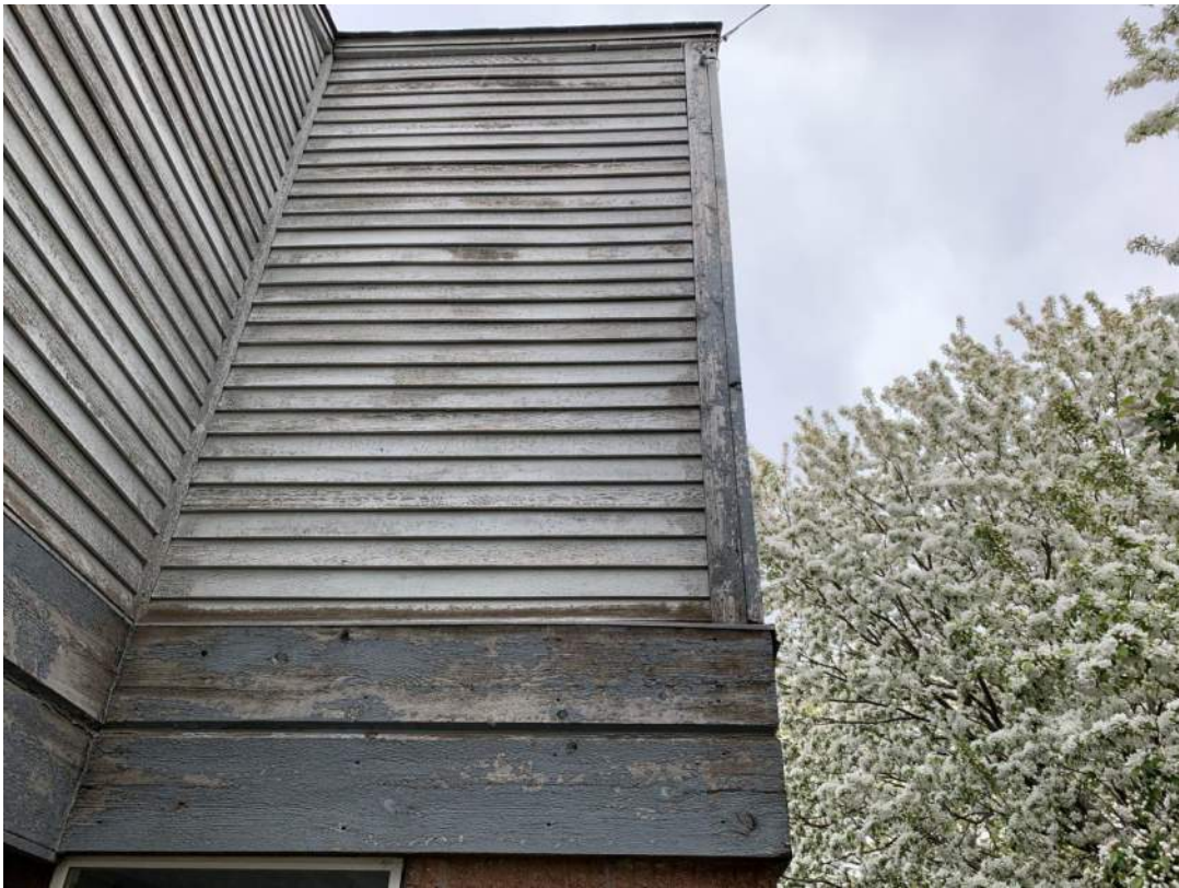
Figure 40 – S34, S35, & S36: SE Side (Gap, Caulking, & Holes)
