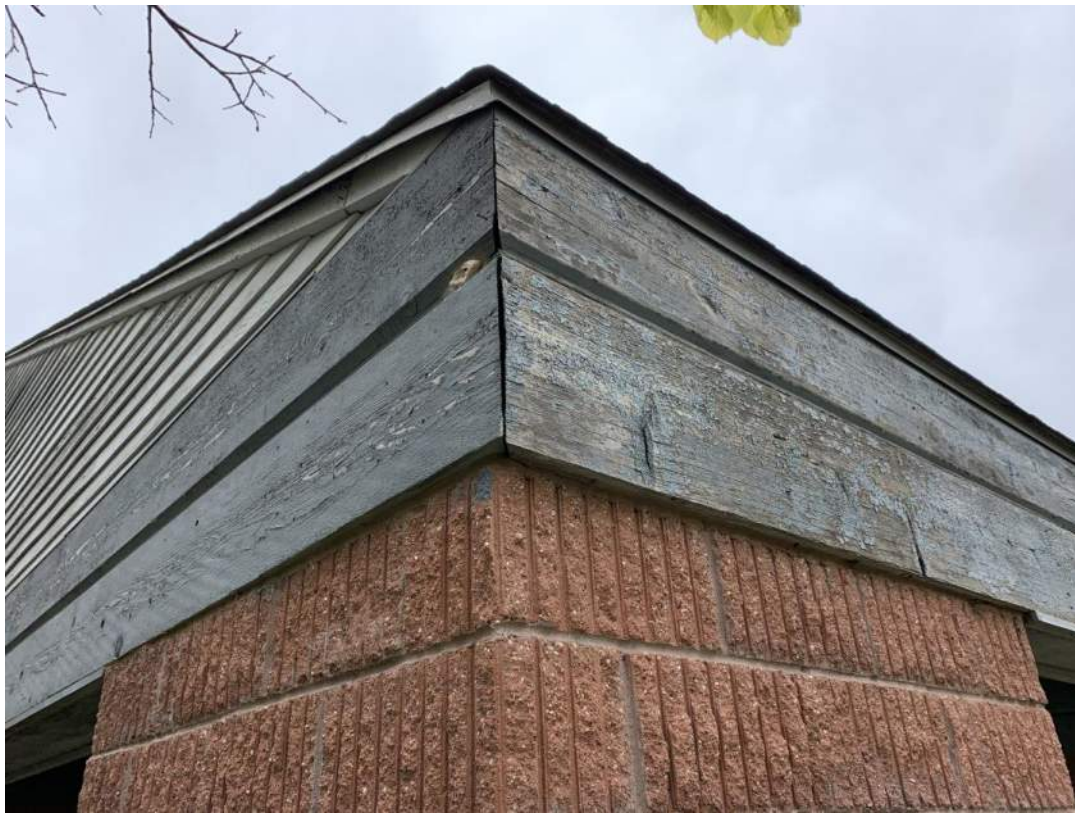
Figure 23 - S18: SW Side (Trim Board Gap)
