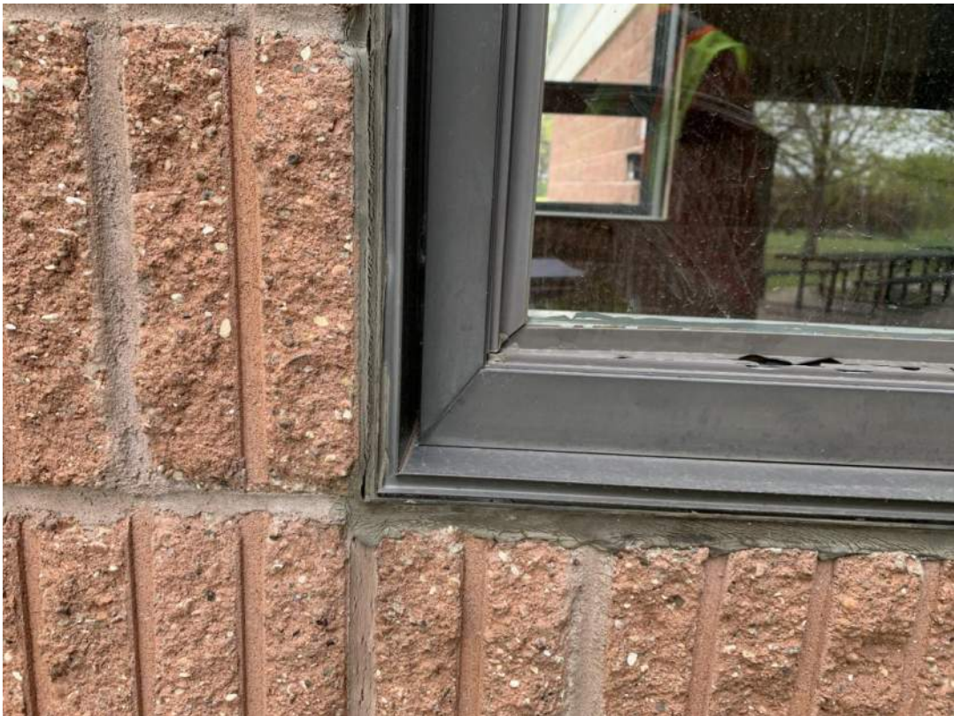
Figure 30 - S26: SW Side (Caulking)
