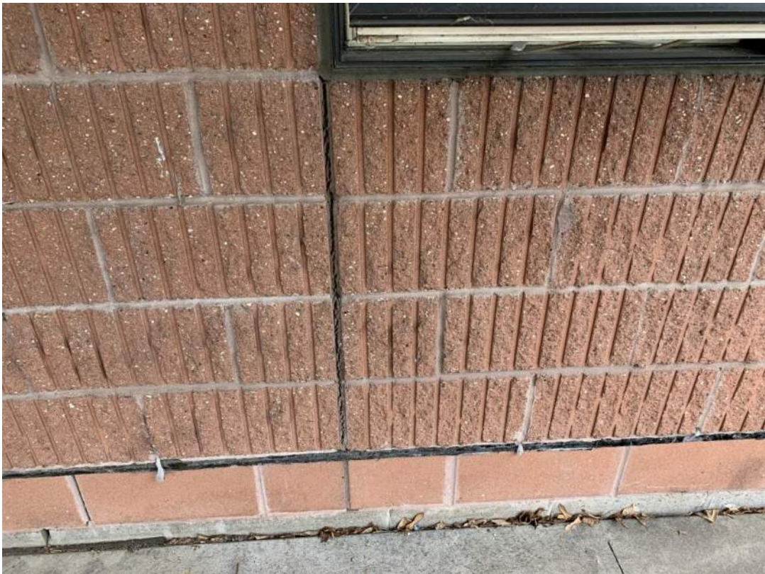
Figure 22 – S17: SW Side (Expansion Joint Caulking)
