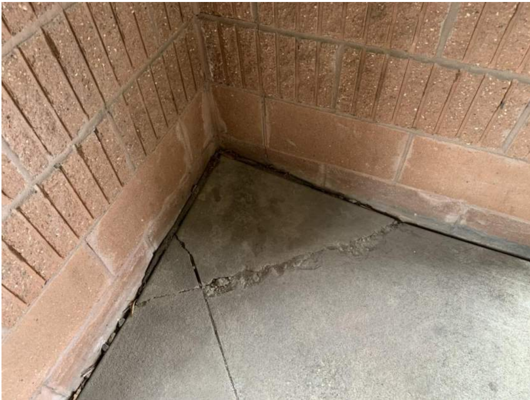
Figure 36 – S32: SW Side (Corner Damage)
