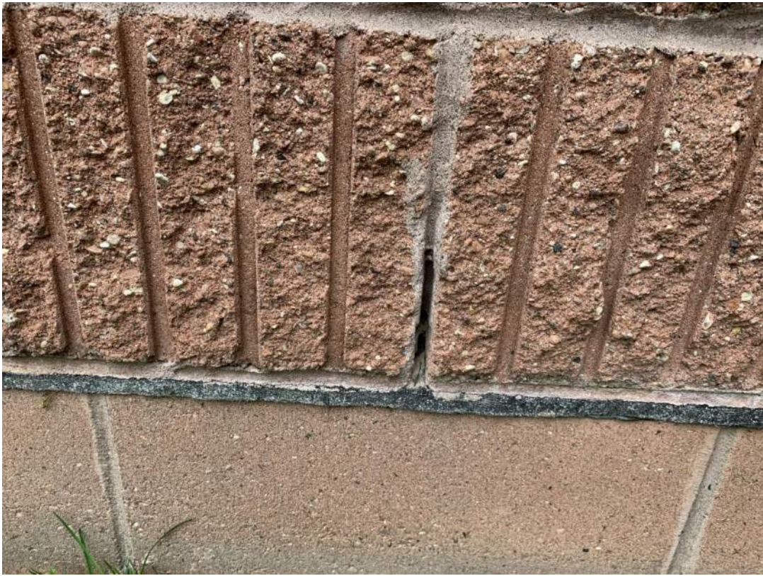
Figure 11 – S3: NW Side (Broken Mortar)
