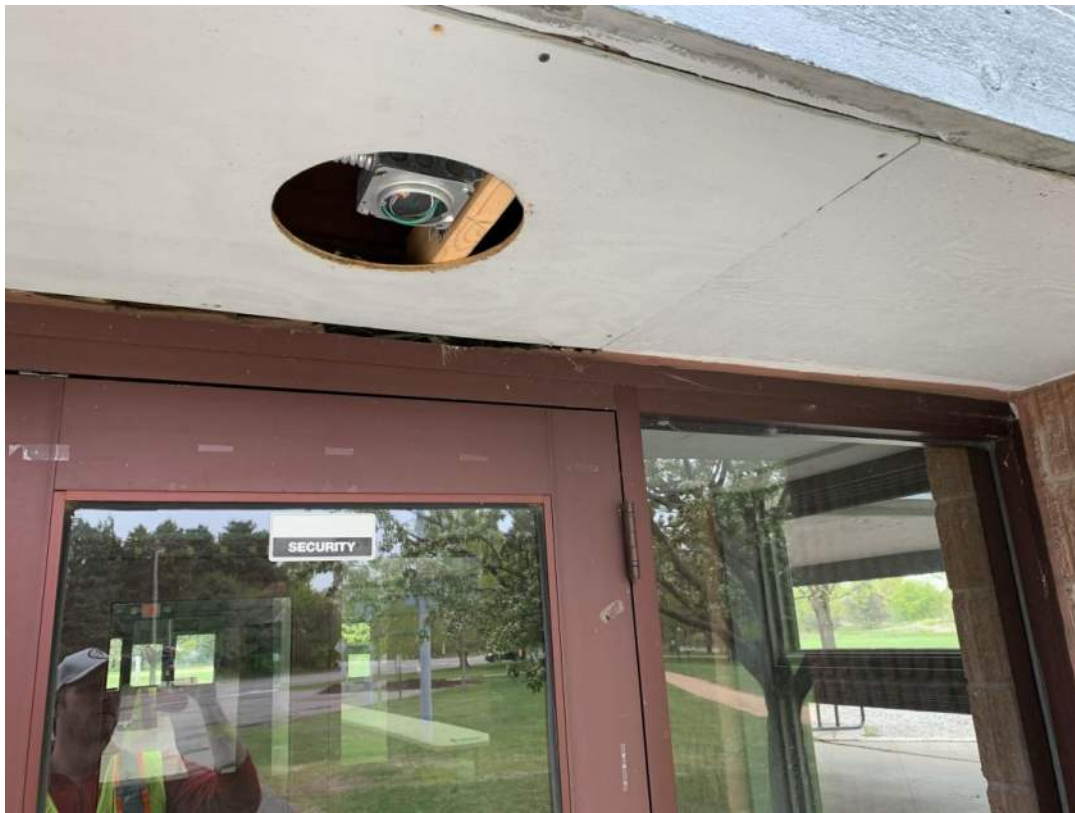
Figure 77 – N1: NW Side (Light Cover Missing)
