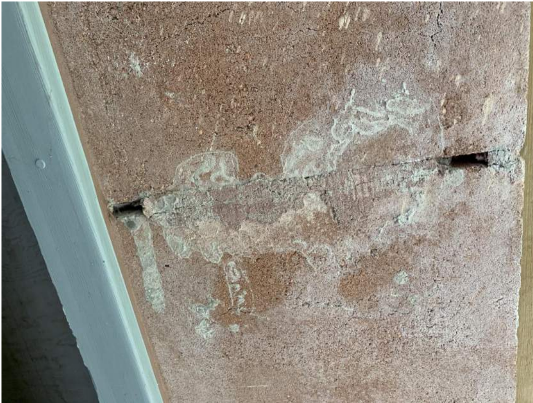
Figure 61 - S56: NE Side (Mortar Breakout)
