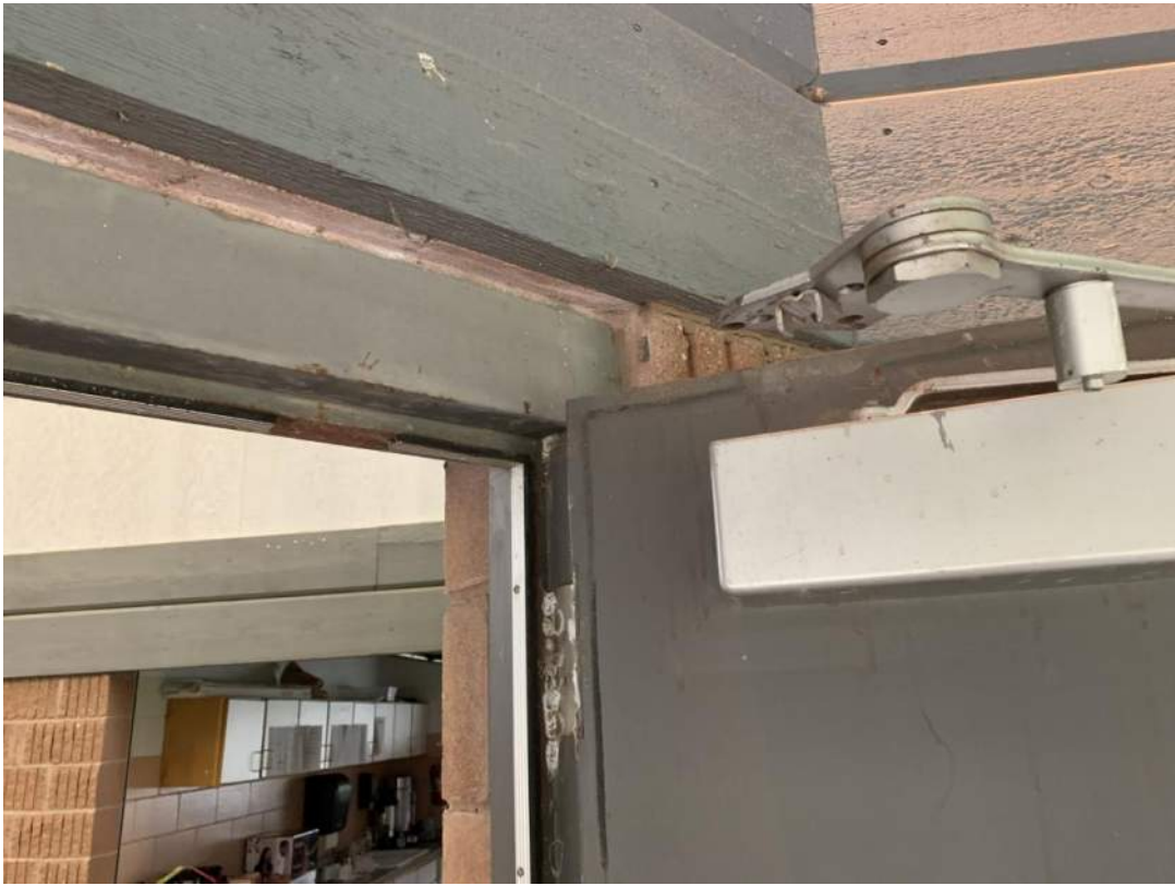
Figure 87 – N11: SW Side (Door Hinge Broken)
