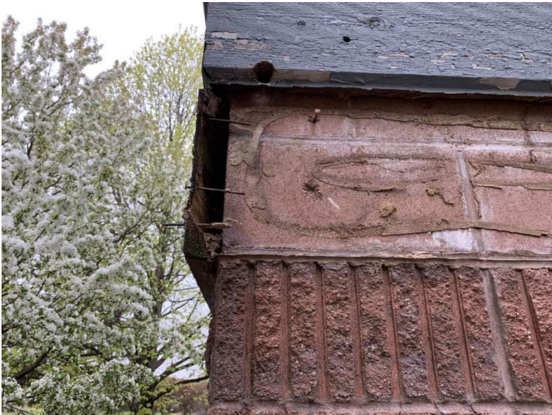
Figure 46 – S41: SE Side (Missing Board & Rotten)
