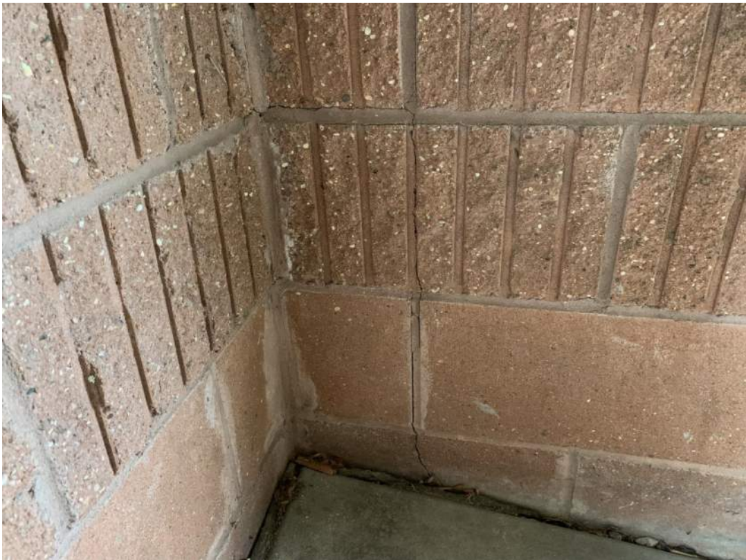
Figure 38 – S33: SW Side (Step Cracking)
