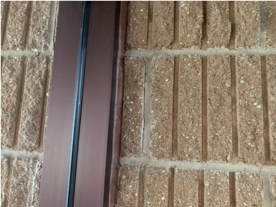
Figure 69 – S65: Main Room (Vestibule Cracks)
