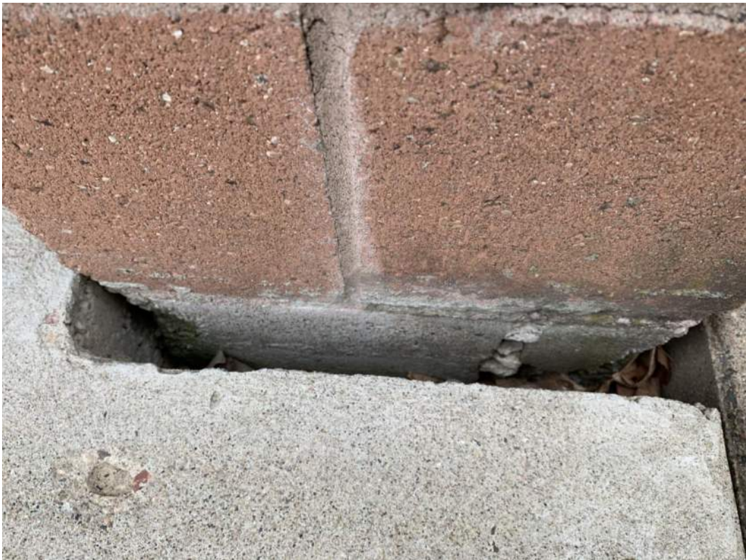
Figure 10 – S3: NW Side (Broken Mortar)
