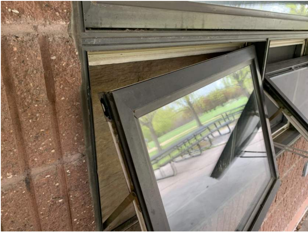
Figure 79 - N3: NW Side (Window Frame Broken)
