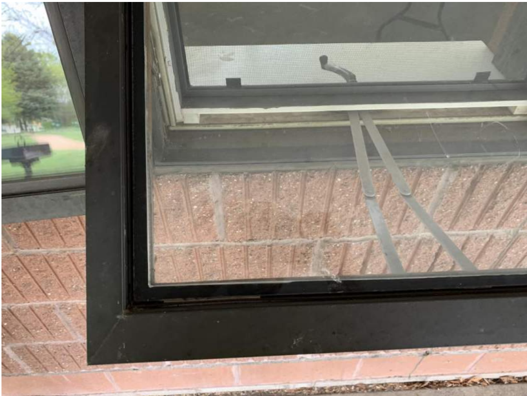
Figure 84 - N8: SW Side (Missing Seal)
