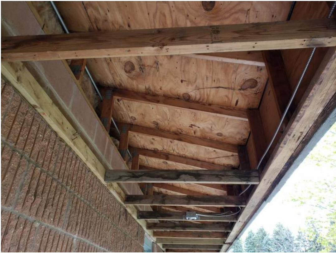
Figure 55 - S49: NE Side (Missing Joist)
