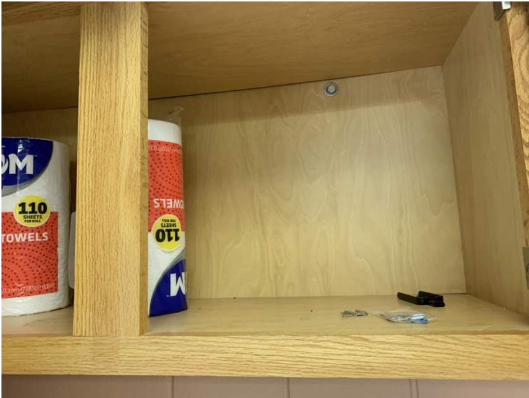
Figure 103 - N27: Kitchen (Cabinet Pulled From Wall)
