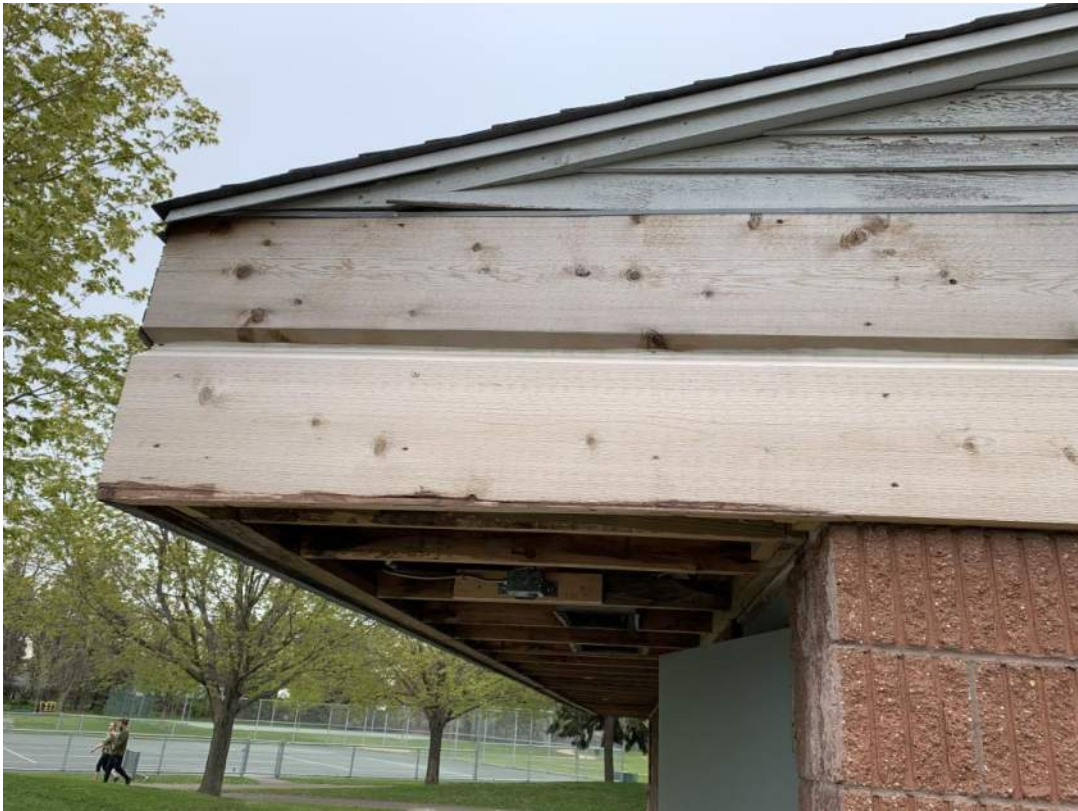
Figure 9 – S2: NW Side (Siding Bowing)
