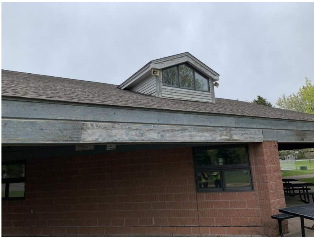
Figure 24 - S19 & S20: SW Side (Water Damage & Paint Flaking)
