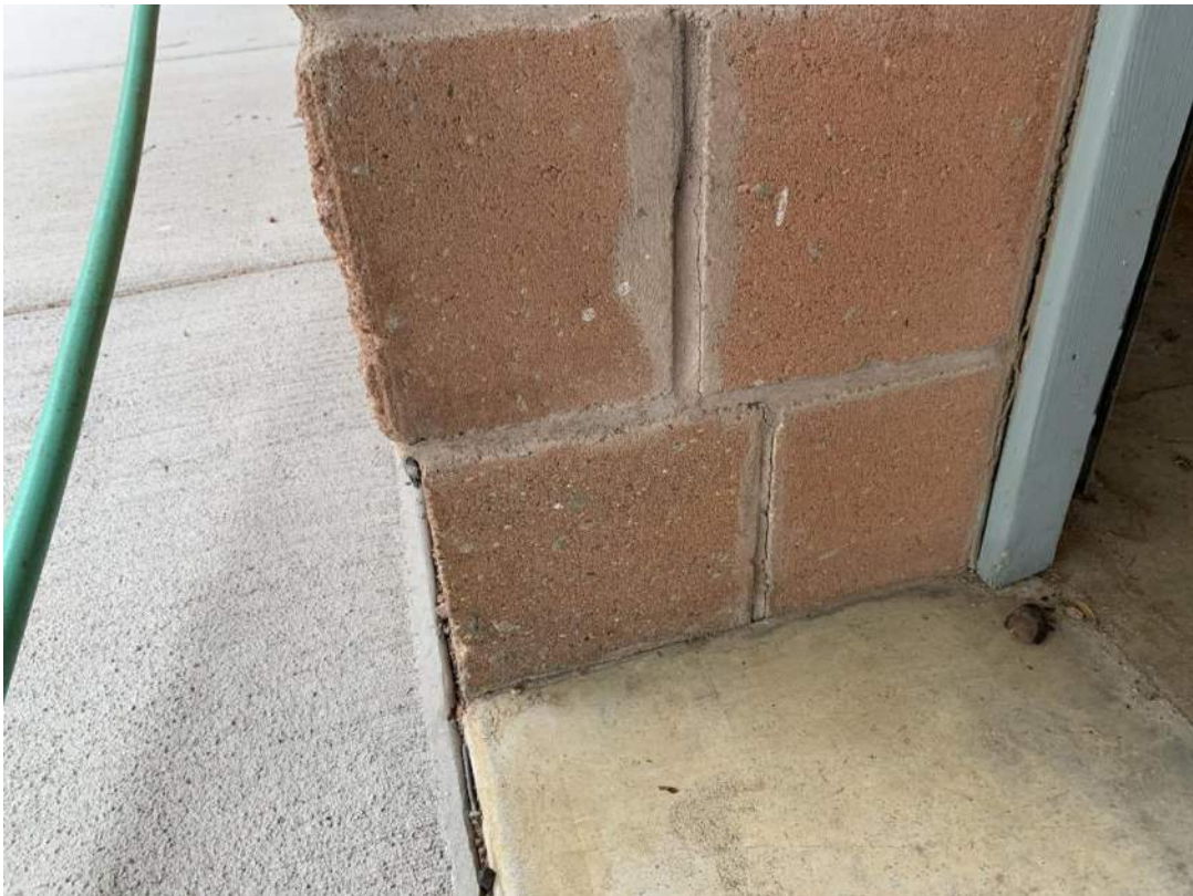
Figure 60 - S54 & S55: NE Side (Garage Door Step Cracking & Caulking)
