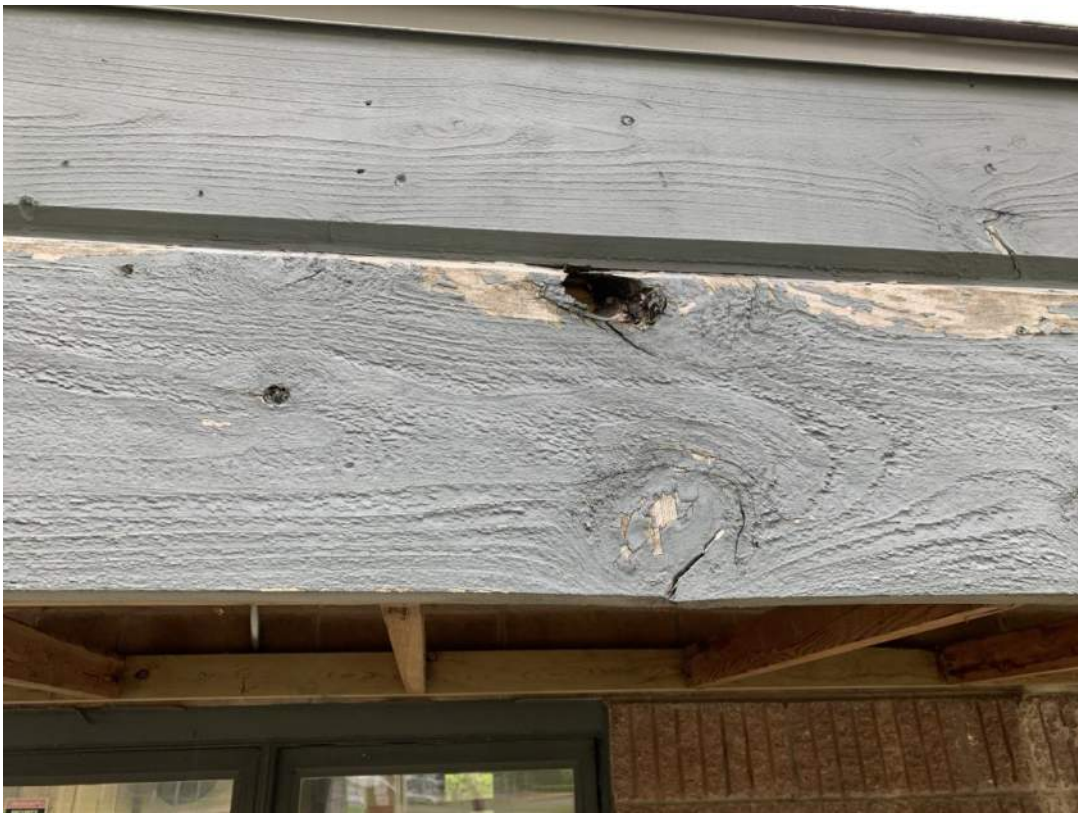
Figure 57 - S51: NE Side (Holes in Trim Boards)
