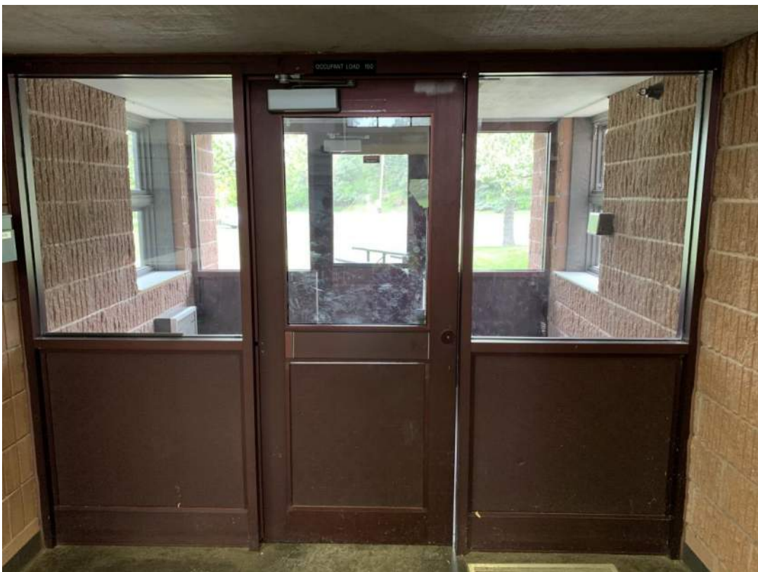
Figure 70 – S66: Main Room (Door Frame Gaps)
