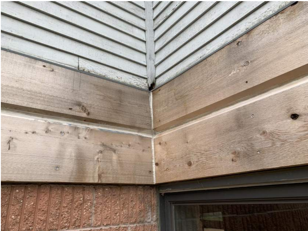
Figure 12 – S4: NW Side (Damaged Siding)
