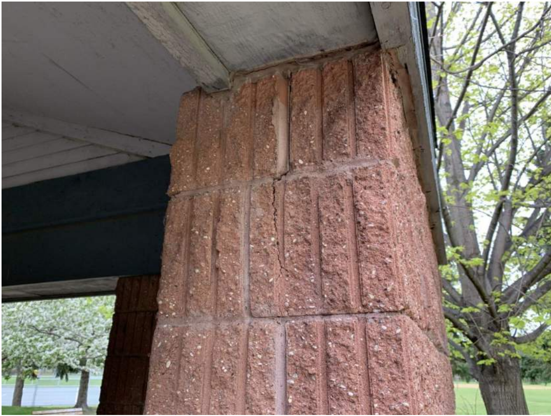
Figure 39 – S33: SW Side (Step Cracking)
