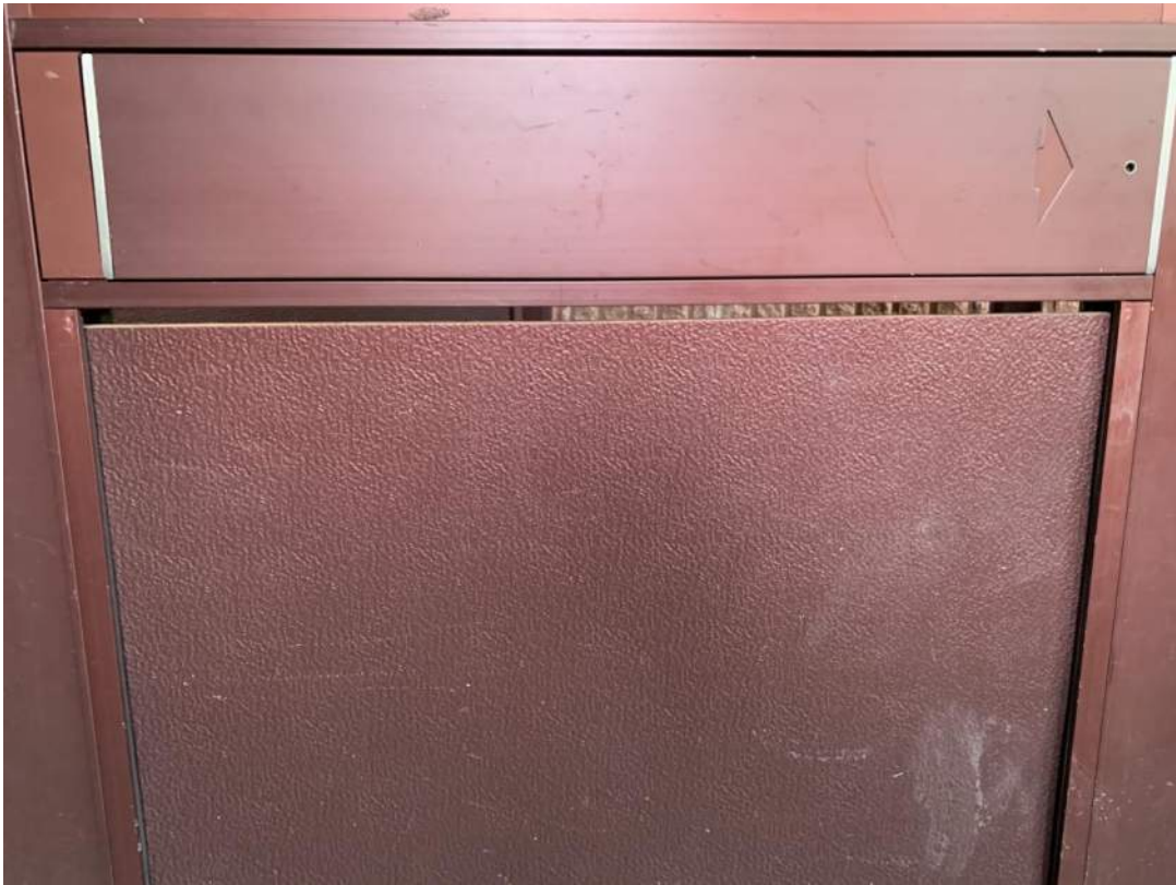
Figure 71 - S66: Main Room (Door Frame Gaps)
