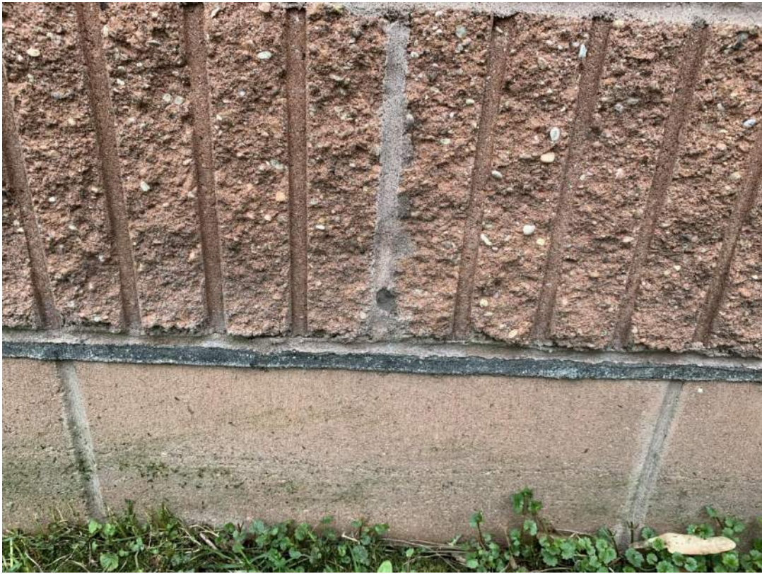
Figure 13 - S5: NW Side (Weep Hole Plugged)
