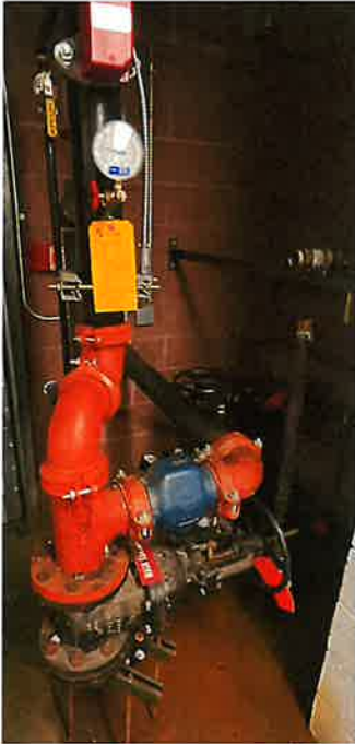
Main Water Service into Building
