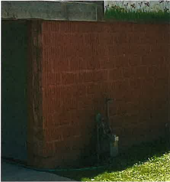
Existing Natural Gas Service.
