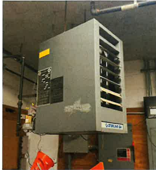
Existing furnaces and unit heater
