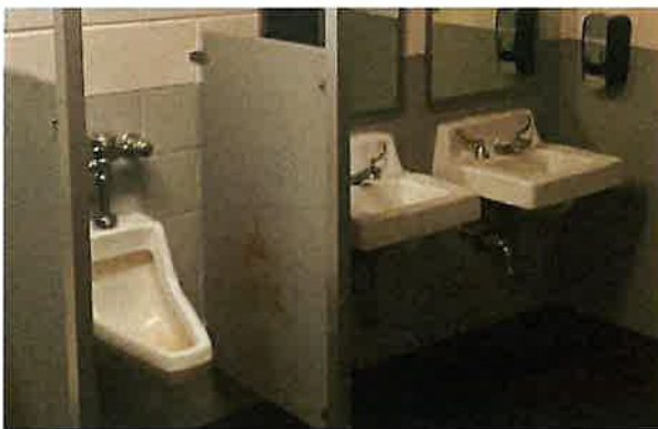
Typical Restroom Plumbing Fixtures
