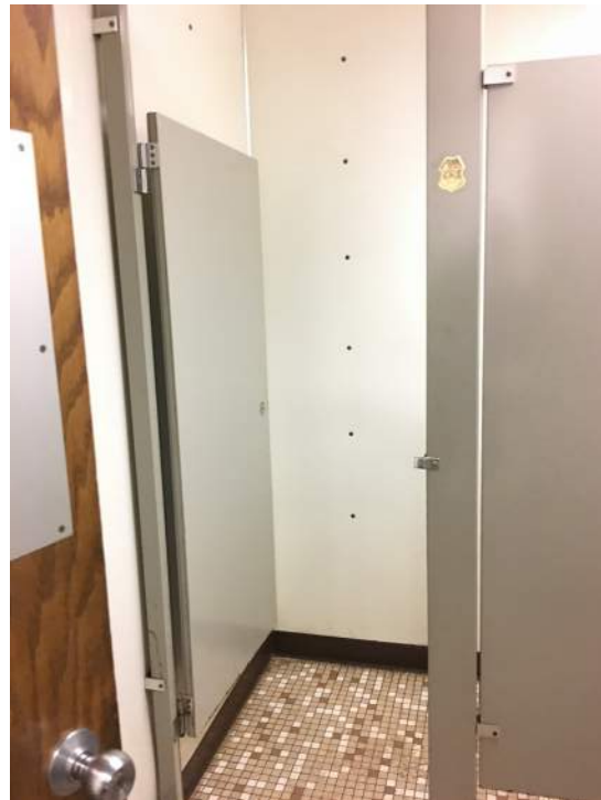
The existing Men's Restroom does not have proper clearances for accessibility, with any amount of remodeling the restrooms would need to comply with the latest Minnesota State accessibility code.
