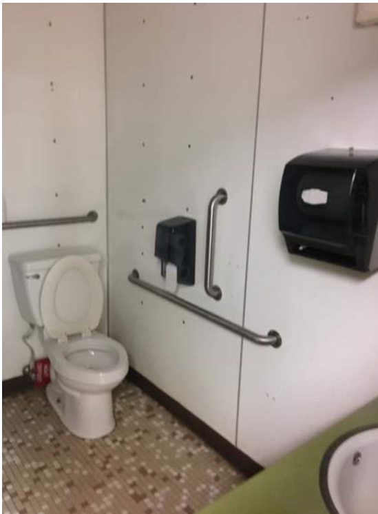
The existing Women's Restroom does not have proper clearances for accessibility, with any amount of remodeling the restrooms would need to comply with the latest Minnesota State accessibility code.
